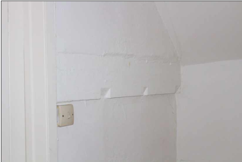
Plate 7: Detail of tie of A-frame truss in landing of first floor dwelling, looking northwest
