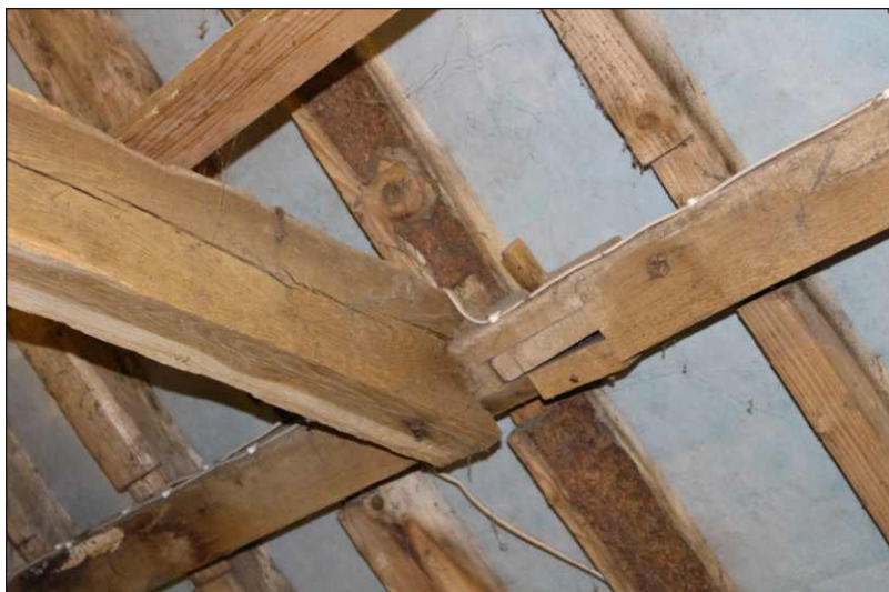
Plate 16: Detail of mortise and tenon joint of south side purlin, looking southeast
