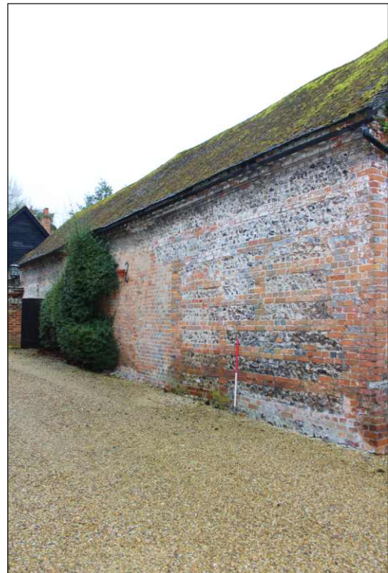
Plate 3: North exterior elevation, showing infilled window, doorway and brick rebuild, looking southeast. (1m scale)
