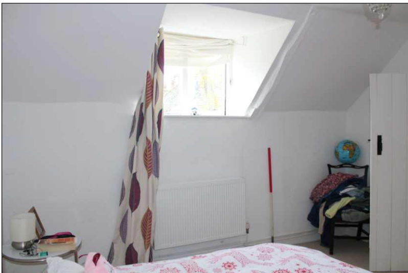
Plate 8: General view of first-floor east room of dwelling showing part of original A-frame truss, looking southeast. (1m scale)
