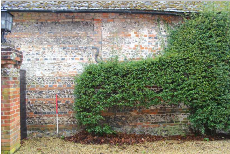
Plate 4: East end of north exterior elevation, showing blocked taking-in door, looking south. (1m scale)
