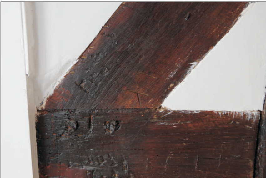
Plate 15: Carpenter's mark on timber framing in the corridor on the first floor, looking east
