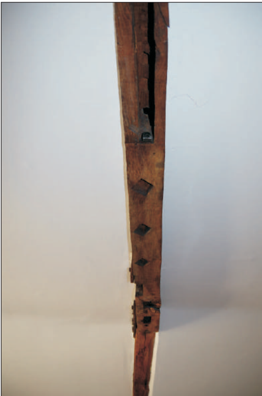
Plate 19: View of empty sockets in base of beam in master bedroom, looking south
