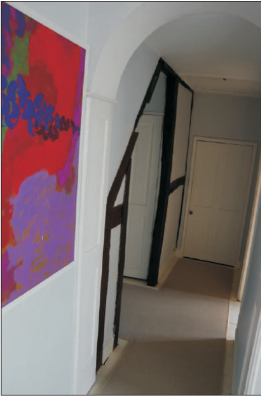
Plate 14: General view of timber framing in corridor on the first floor, looking southeast
