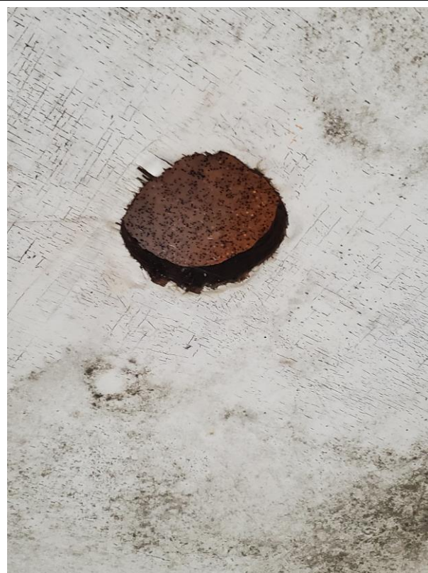
Interior hole in ceiling
