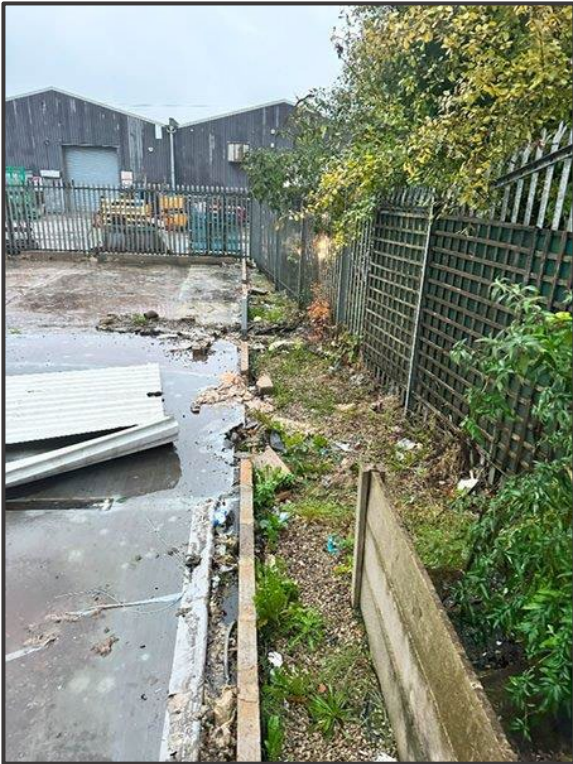
Picture 1. Foundation and heavily compacted hardstanding has likely deflected roots from T1 & T3.
