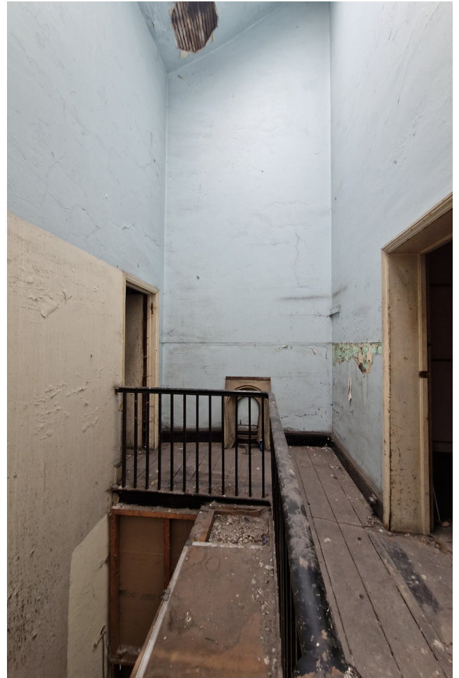
Existing condition of the communal central stairway. This condition follows right to the ground floor.
