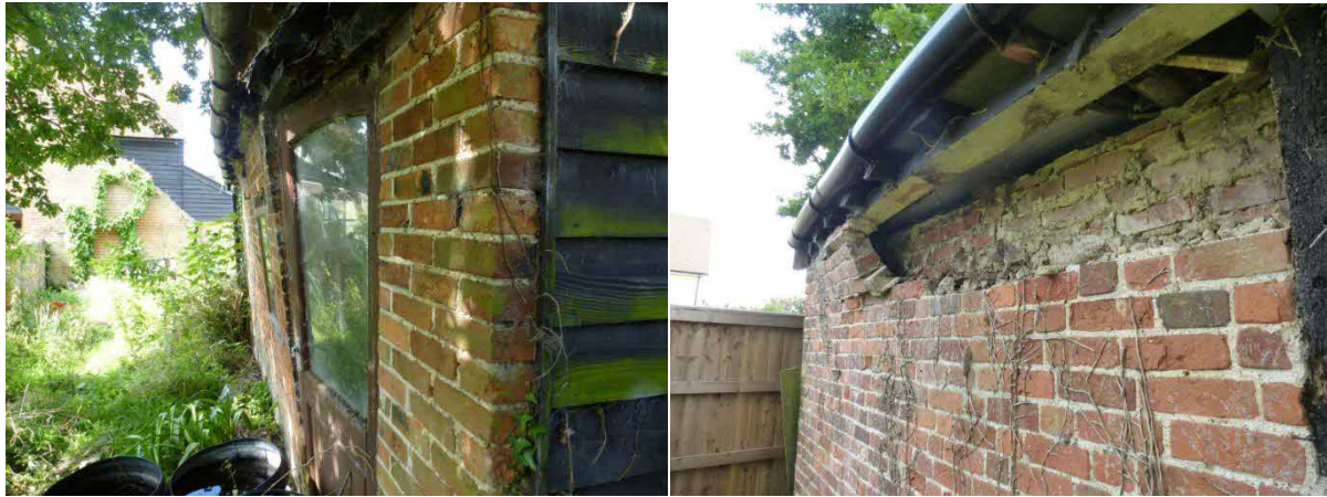
Figure 18, left: The leaning wall of the shed following the collapse of the roof Figure 19, right: the outer skin of brickwork partially collapsed after the roof fell in, exposing the inner skin of brickwork.
