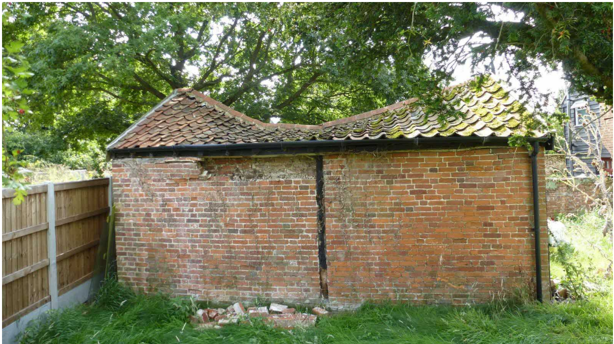
Figure 17: photograph of the old shed in 2014 with its roof partly collapsed
