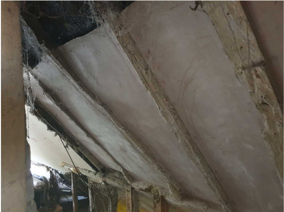
Figure 16 Two of these undersized rafters would need to be removed to create head height; allowing the stairs to be used safely. The tiny knee braces suggest that they have been retro-fitted. They would be recorded before removal
