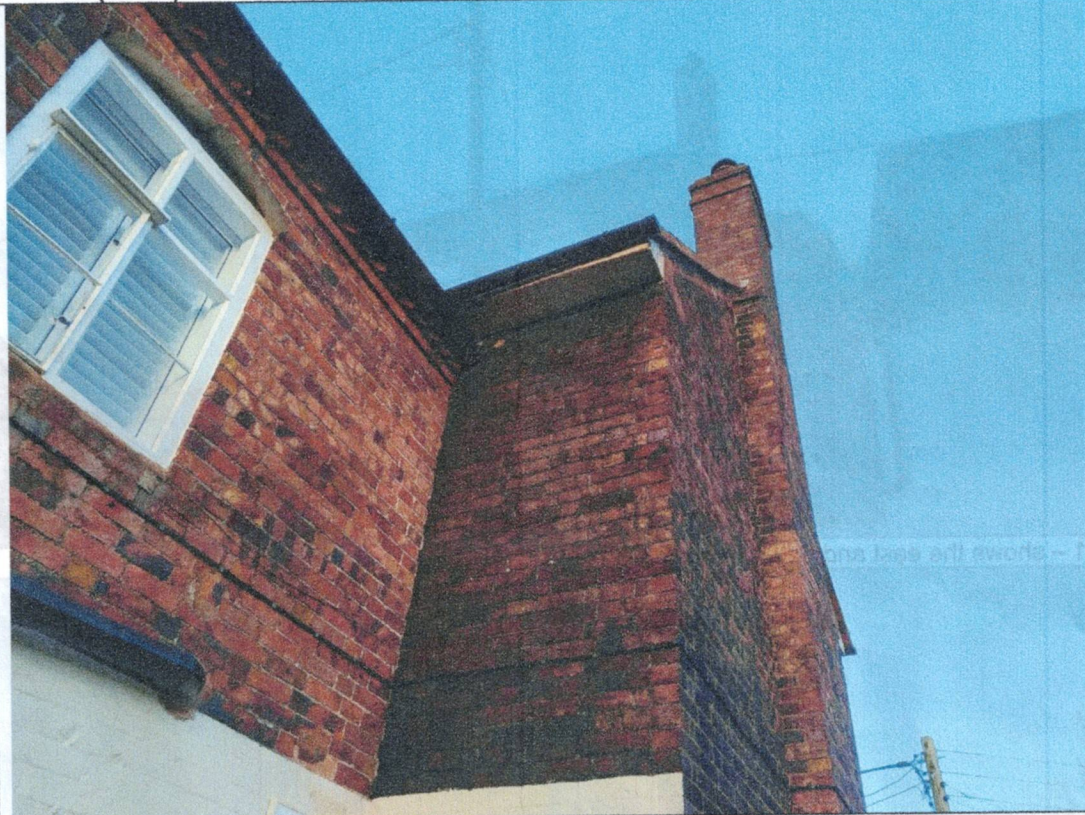
Photo 3 – shows the south-facing elevation with an example of the recently replaced and thus tightly fitting soffits
