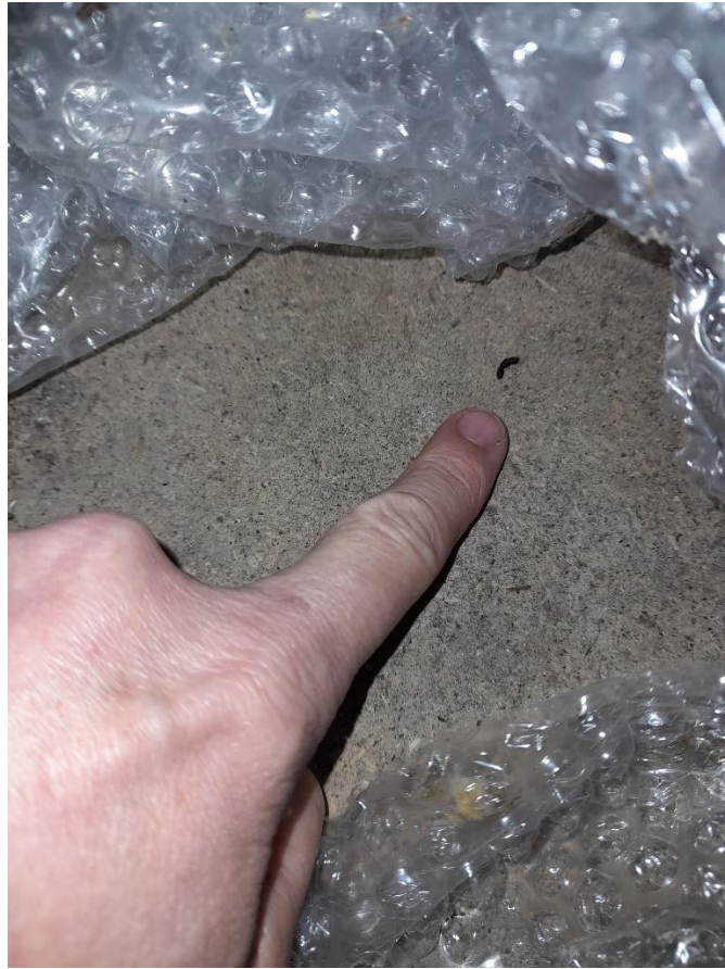
Photograph 8: Evidence of a bat dropping within the roof void.
