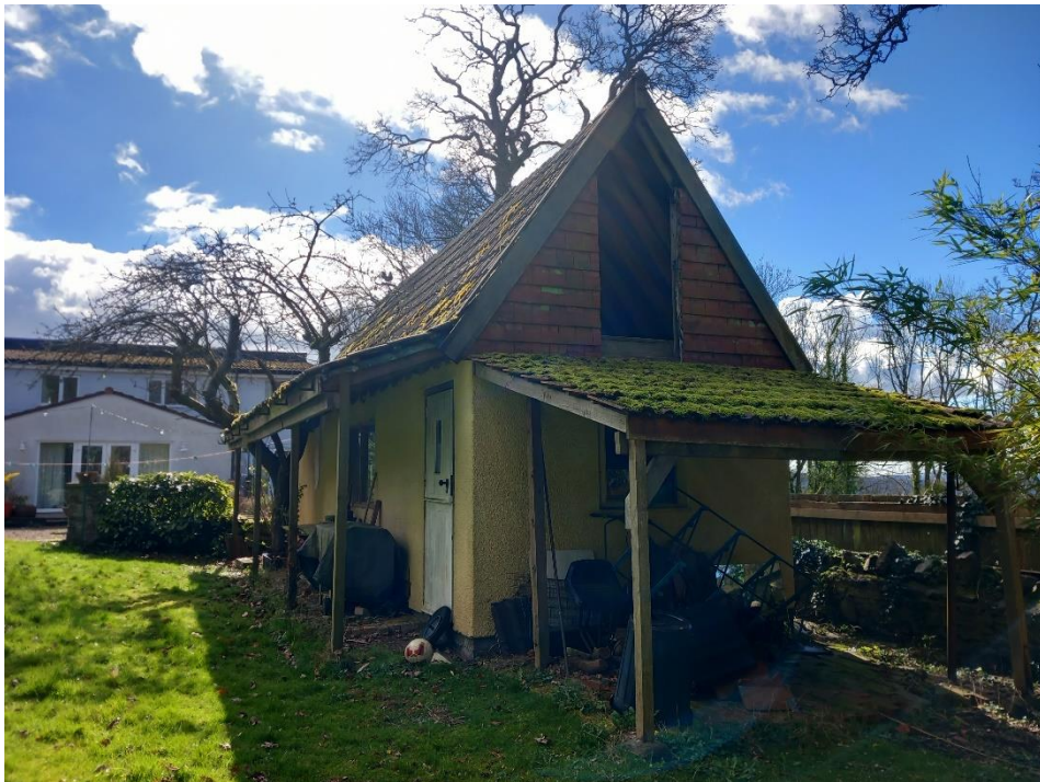
Photograph 1: Northern aspect of the garage showing the lean to and access into the roof void via the open doorway above.
