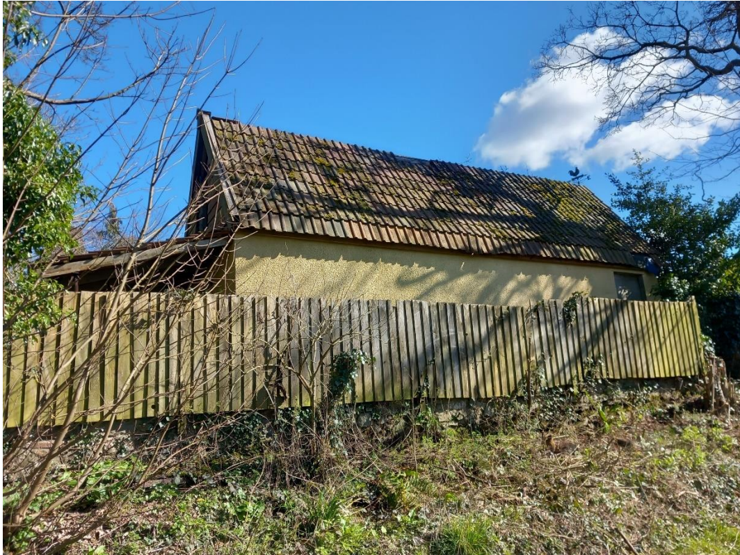
Photograph 4: Western aspect of the garage. Single ridge tile present at the northern end and missing tiles present below the ridge in the centre of the roof and in the southern corner at the bottom of the roof.
