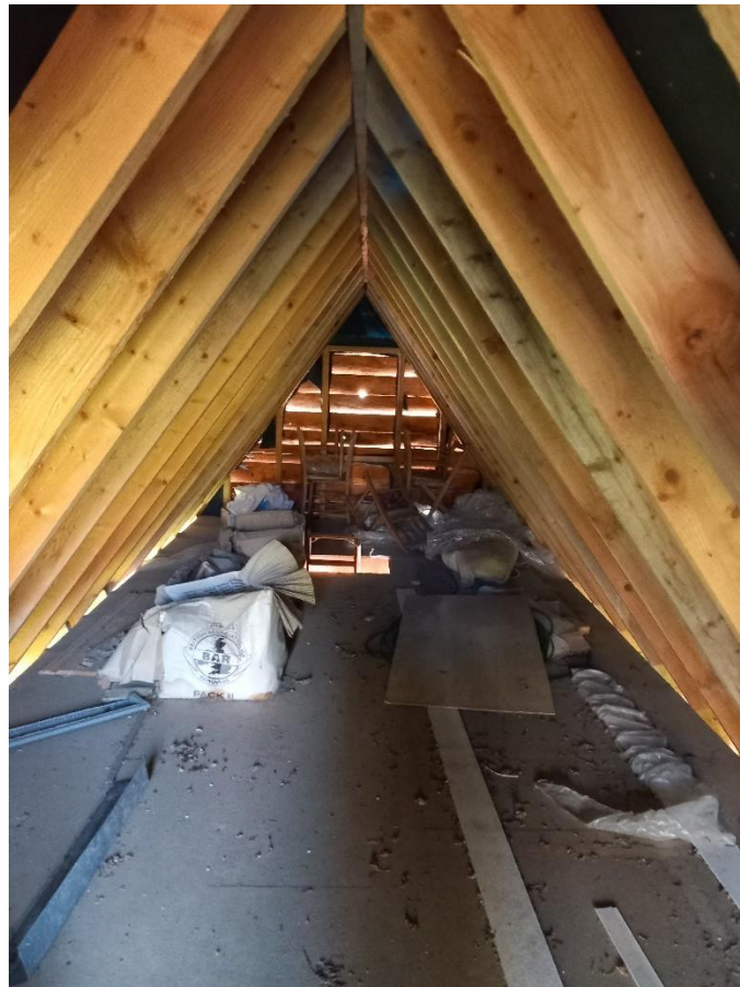
Photograph 7: Gaps in wooden cladding at southern end of the roof void.
