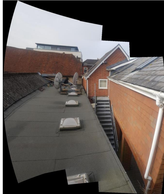
Flat roof to corridor showing Building in Gables Yard to North of corridor
