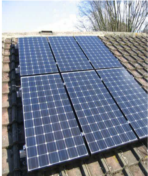
Figure 7 - Photovoltaic array on a pitched roof
