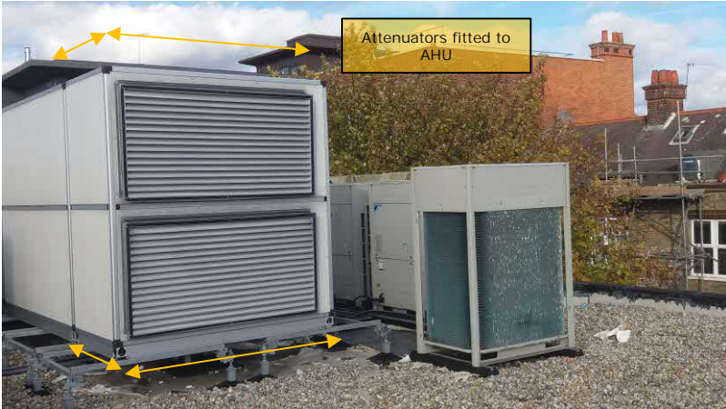
6: Existing plant from south
