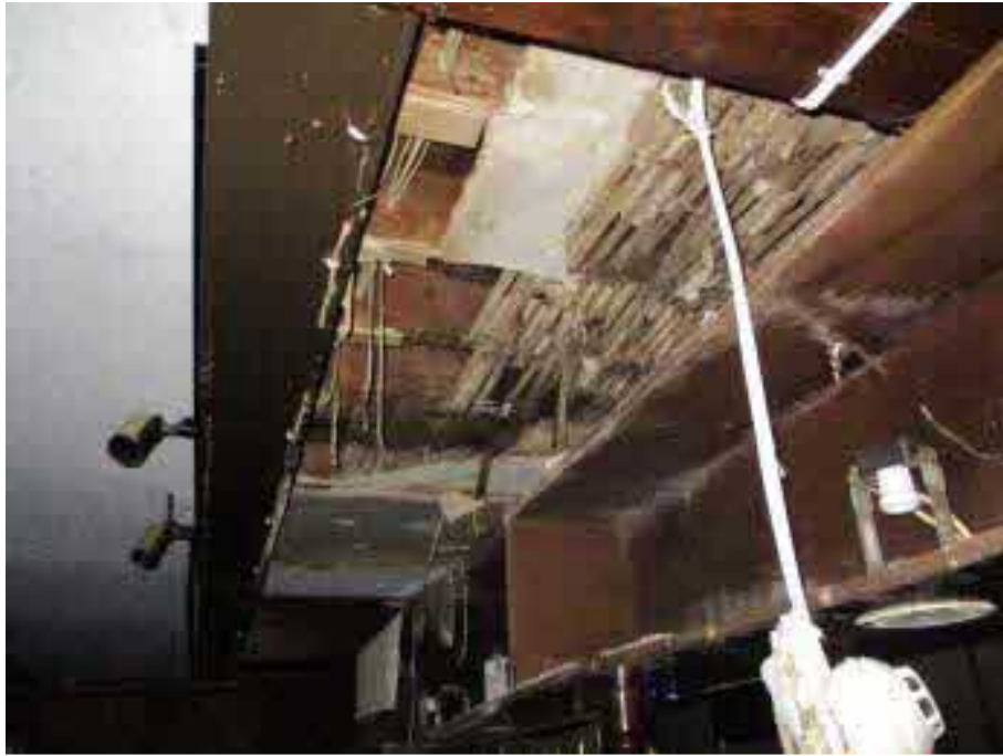
Water damaged ceiling above bar
