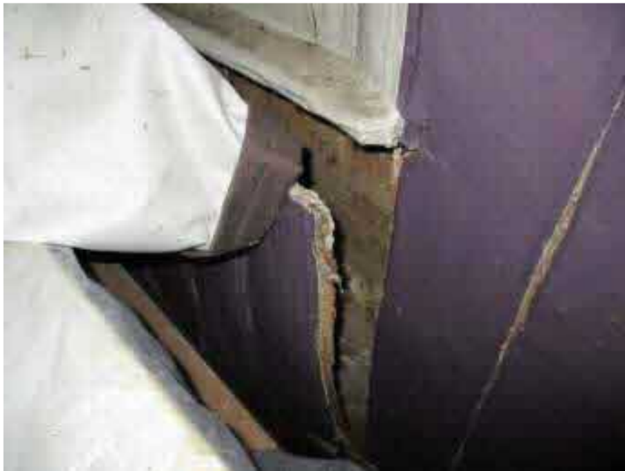
Damaged panelling in bar area
