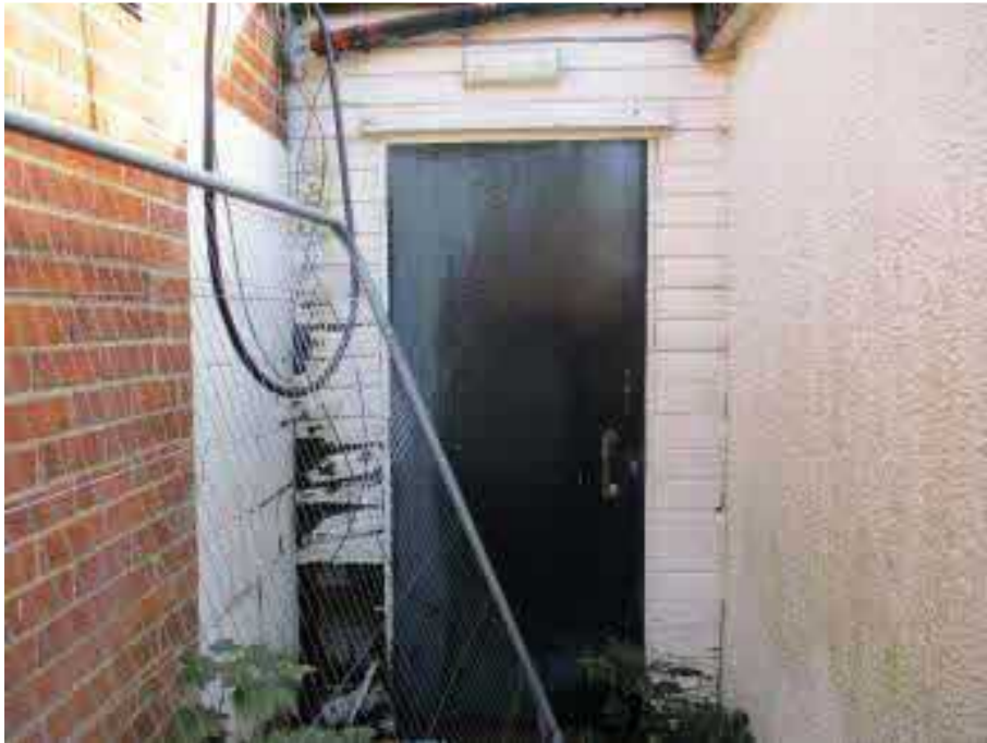
Rotten side entrance
