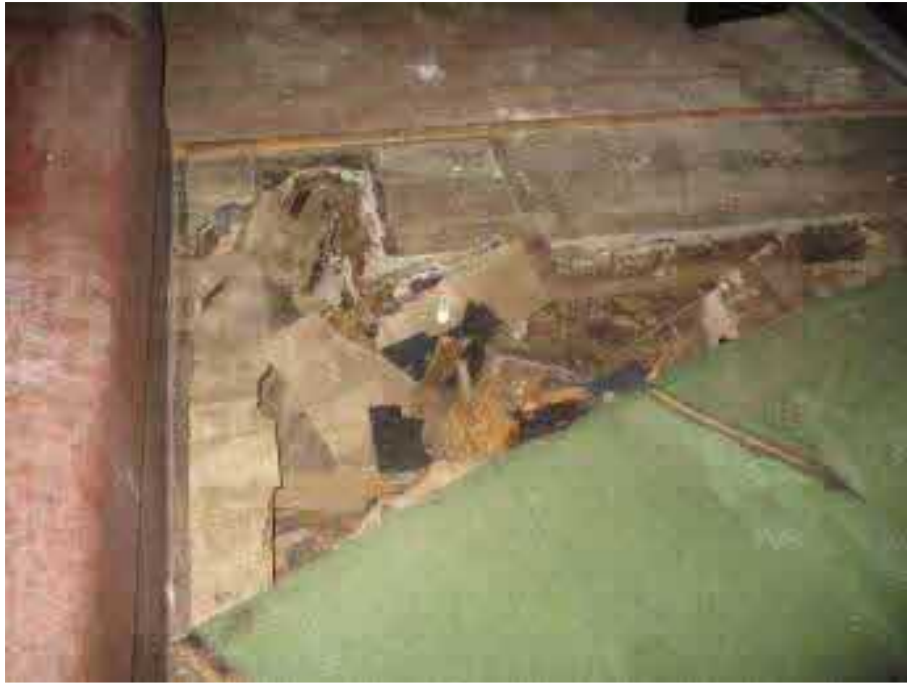
Collapsed bar floor
