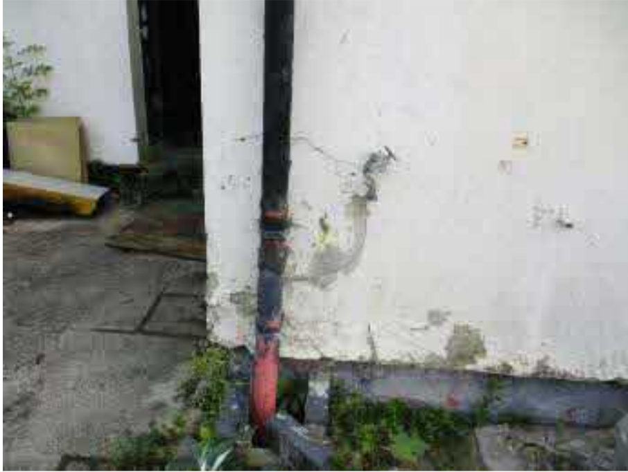
Blocked and leaking downpipe and loose render
