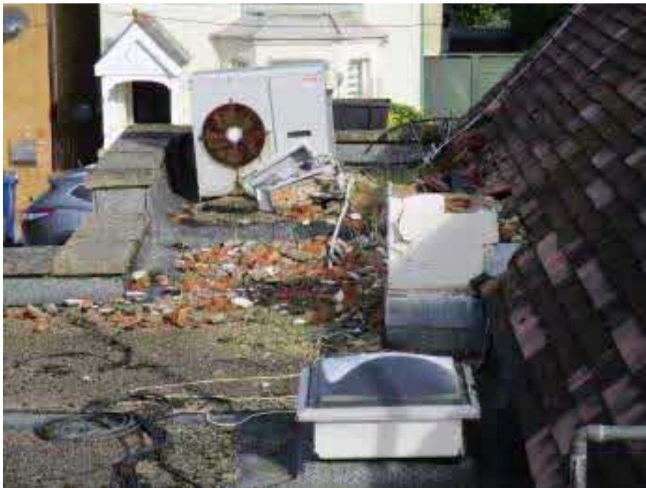
Collapsed chimney on flat roof
