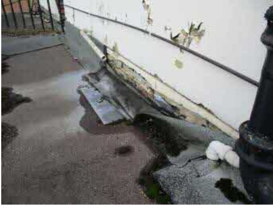
Flashing pulled away
