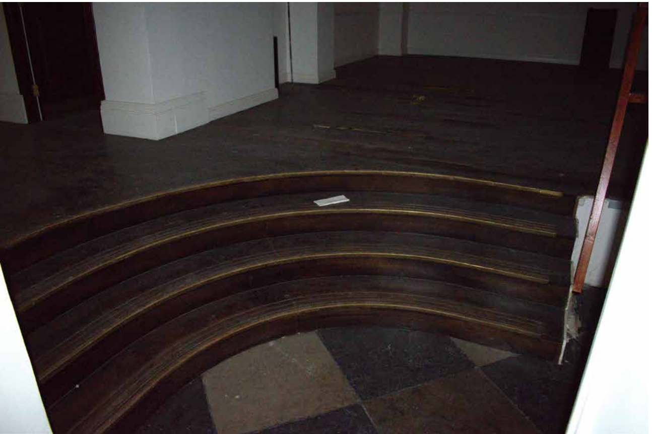
Plate 13 Detail showing raised timber floor to north side of ground floor (DIA)
