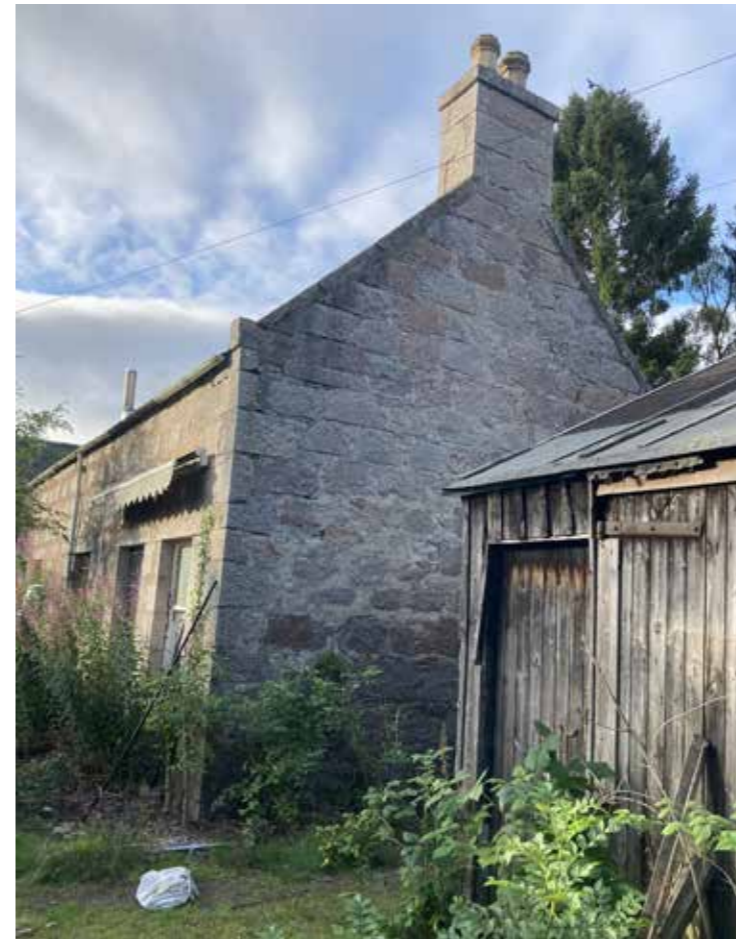
1. Photograph of inner courtyard showing dilapidated garage
