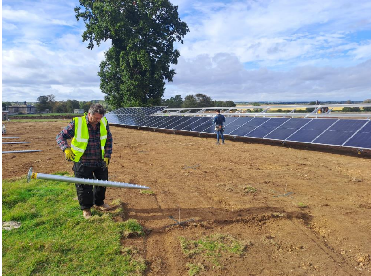
Figure 3: A Ground Screw Shown for Scale with Panel Arrays in the Background
