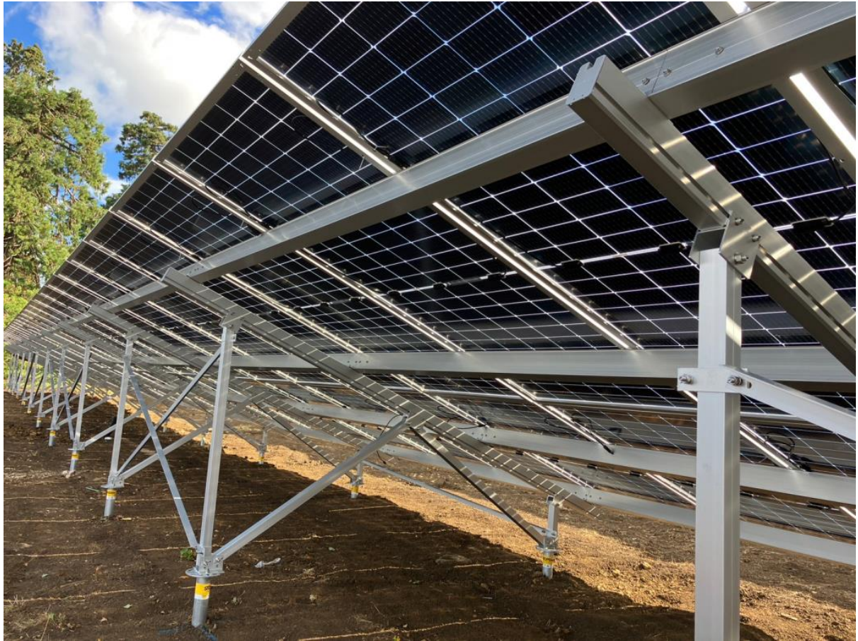
Figure 6: View of the light-collecting underside face of an array of panels installed at the Lilford Hall site
