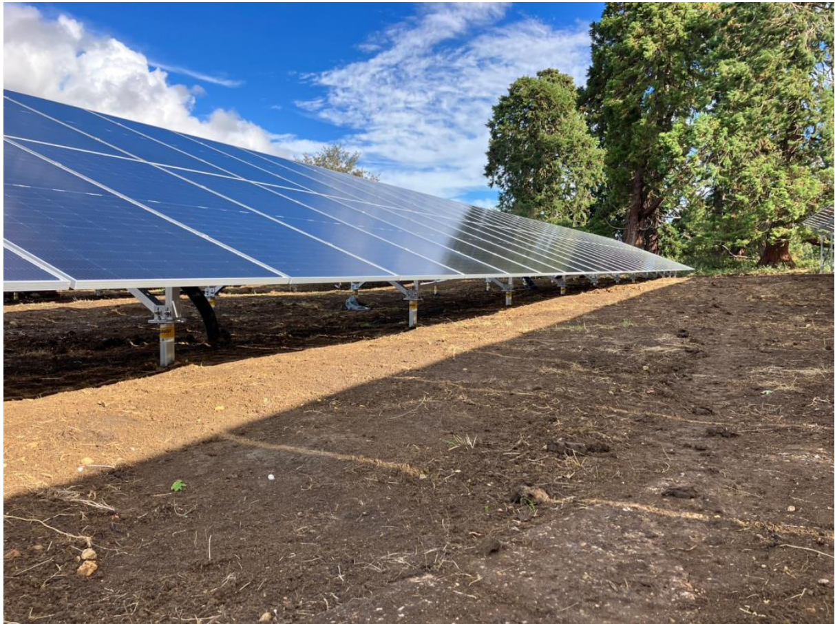
Figure 5: Top view of an array of panels installed at the Lilford Hall site
