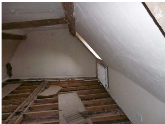
Bed 6 requiring new floor
