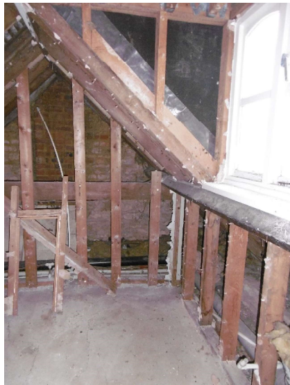
Dormer to be removed and bathroom to be returned to roof space
