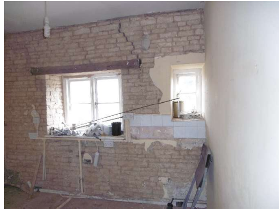
Laundry with modern window to be removed
