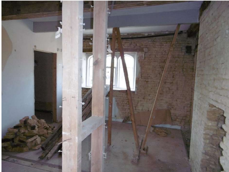
Bedroom 1 with structural issues
