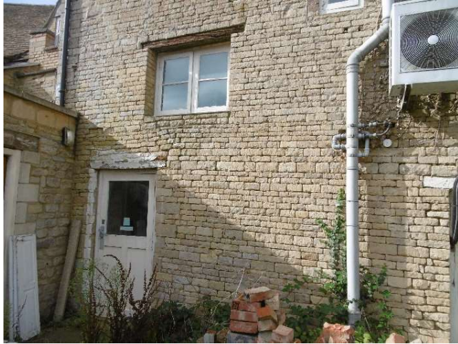
Back door to be replaced and showing Movement in masonry
