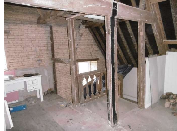
Crack showing at high level internally
