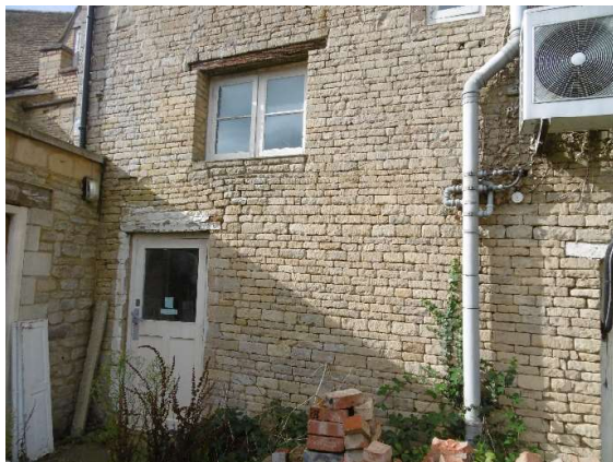
Movement on rear gable
