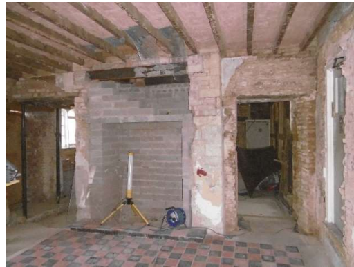
New snug: Reinstatement entrance lobby by front door, form new fireplace, block up single door openings, new plasterboard ceiling
