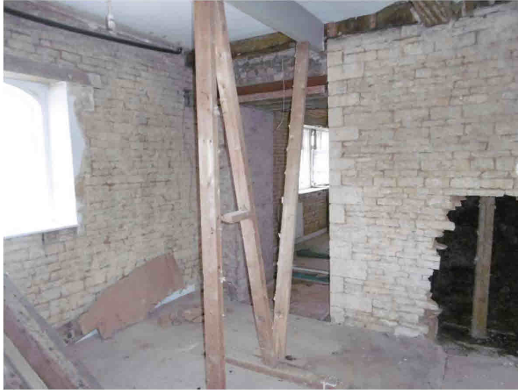
X20 with missing bearing,
