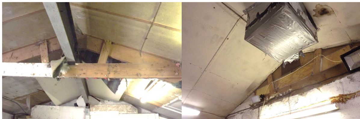
Fig 7. Internal view of roof structure and sealed up vents
