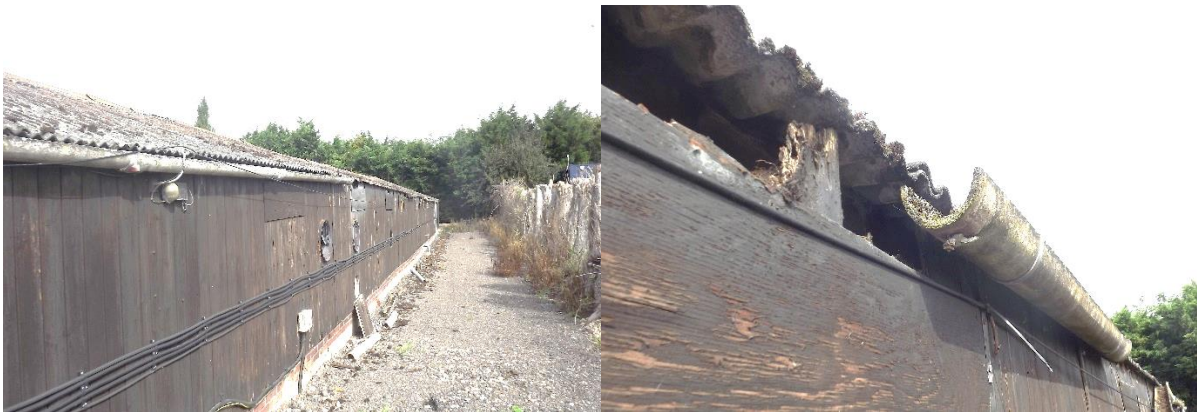
Fig 6. East elevation (left), rotten timbers and broken roof sheets (right)
