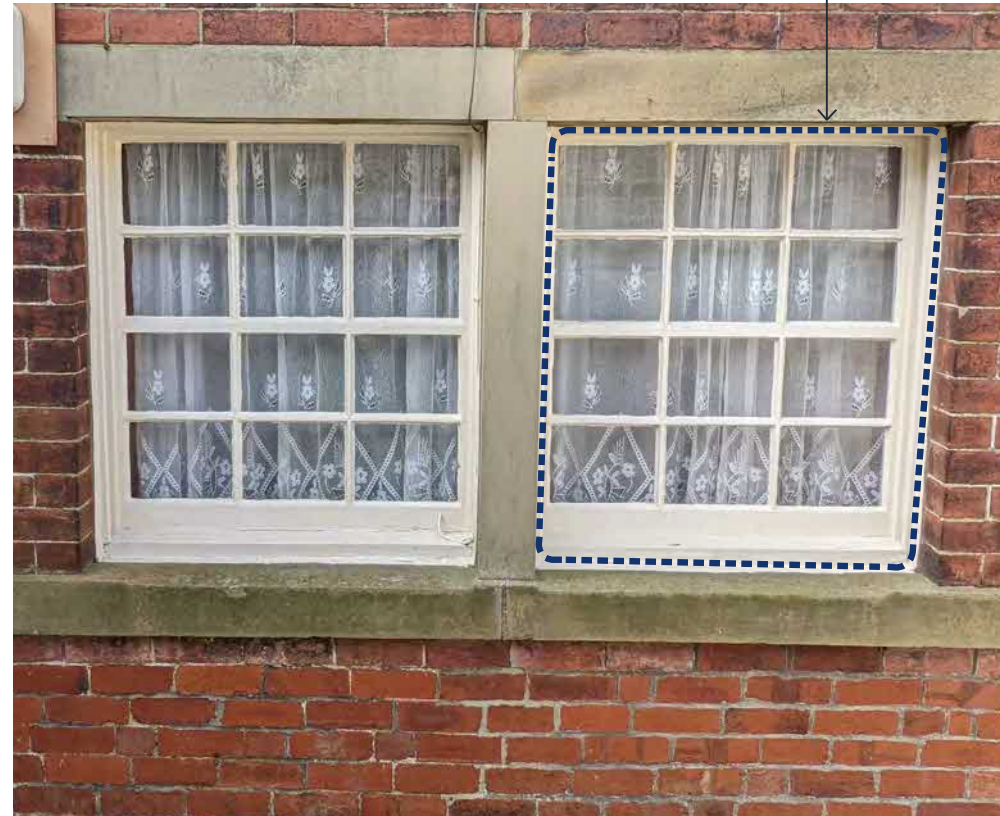
Typical example of a pair of sliding sash windows with stone pillar between, stone cill and lintel (located within octagonal bay at front / east elevation of main building)
