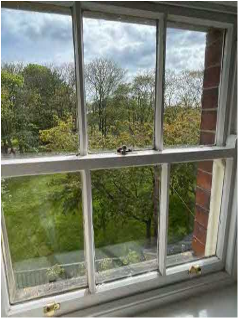
Detail of typical window unit showing glazing bars and hardware including sash locks and pull lifts
