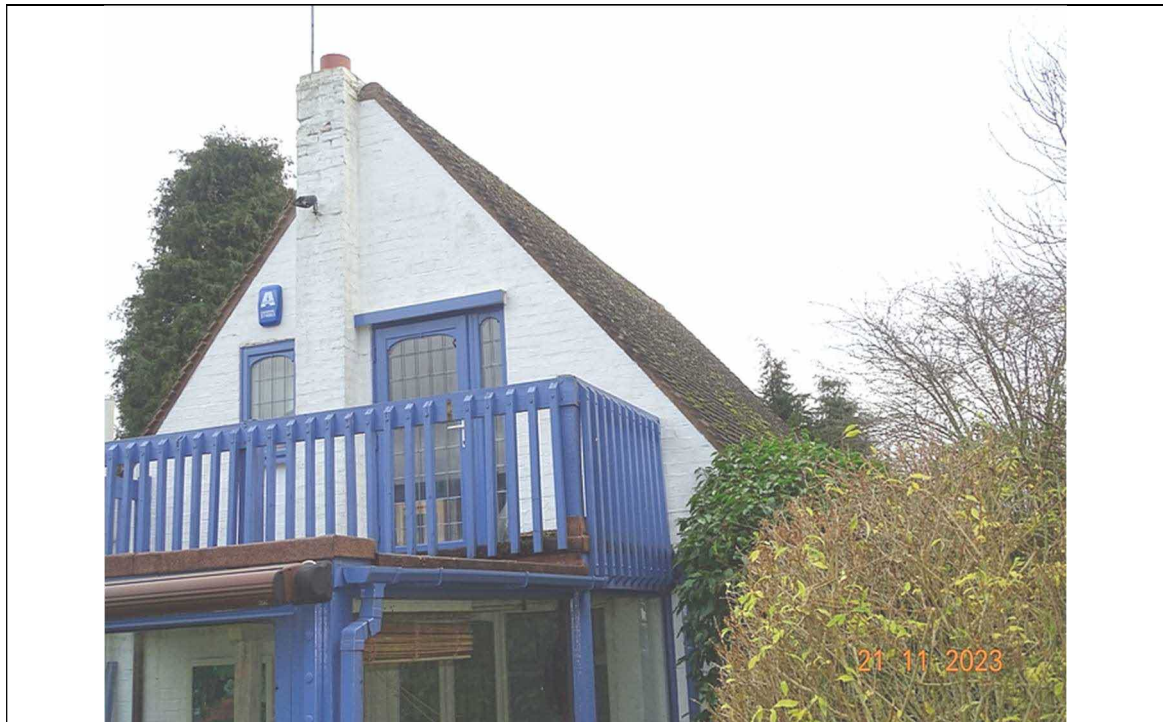
Plate 5 | Describing west gable and looking along south facing roof of cottage from CP(E)
