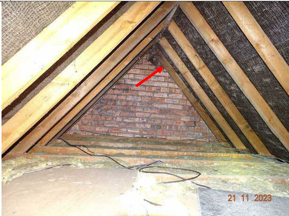
Plate 8 | Looking along loft towards western gable wall. Arrow indicates gap where light was visible, leading to loose flashing around part of chimney.
