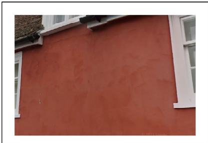
Render starting to crack around window frames and under dormer at the eaves.
