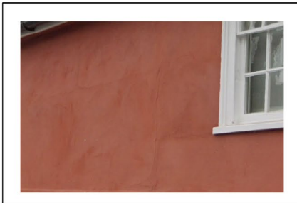
Render starting to crack around window frames
