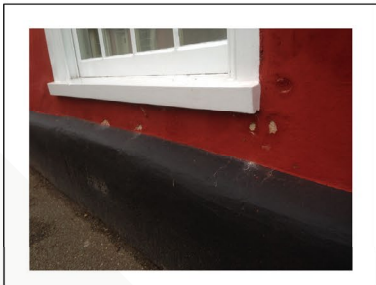
Noticeable damage to render under cill which will be repaired by proposal
