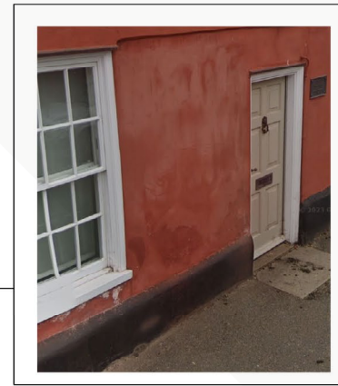
Paint fading and staining brick plinth caused by badly draining gully. To be repaired
