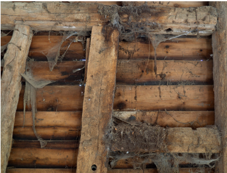
Fig.3 Evidence of a previous mullioned window with sliding shutter in Old Rectory Barn
