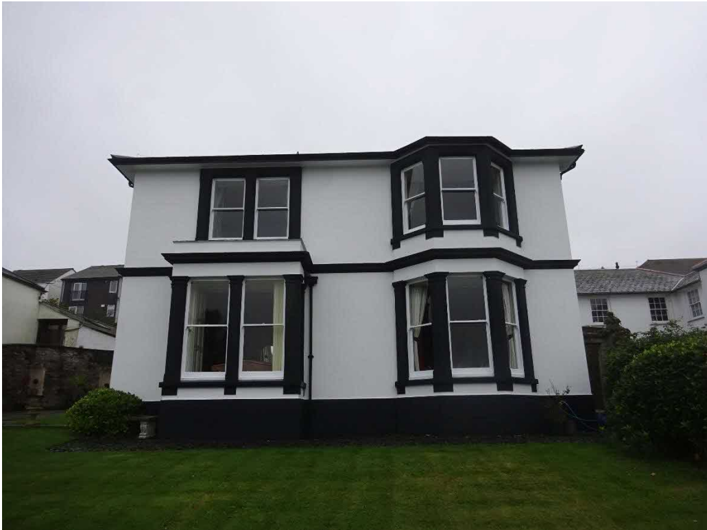
North East elevation as seen from within site boundary. Stratton Terrace is at a lower level. Note; Limited visibility of roof coverings from Stratton Terrace and therefore the proposed bird protection system has limited impact.
