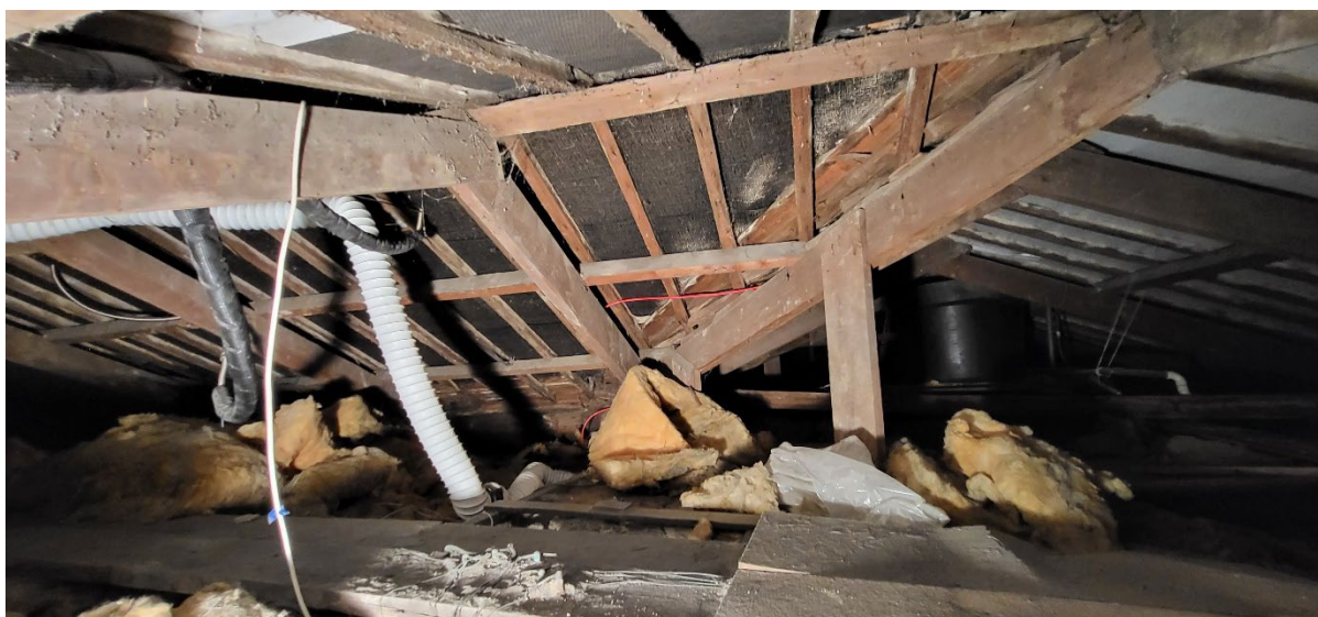
Figure 9: Internal structure of the roof void. Timber frame and slates lined partly with bitumen roofing felt and partly a breathable membrane
