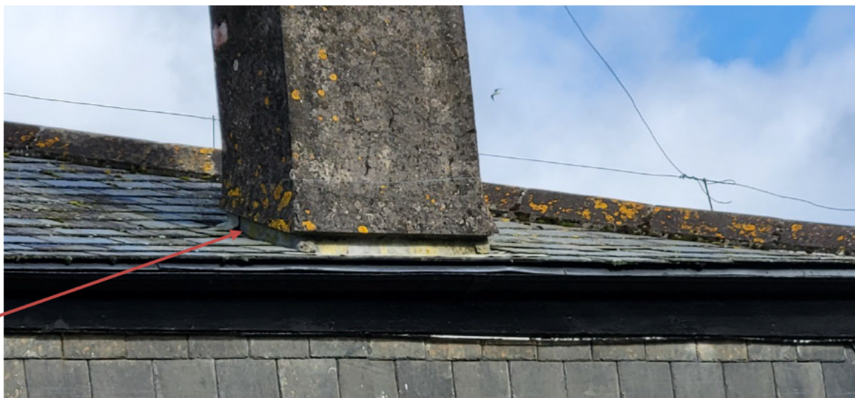
Figure 3: Crevice beneath lead flashing at the base of the chimney on the West elevation may provide an access point for roosting bats
