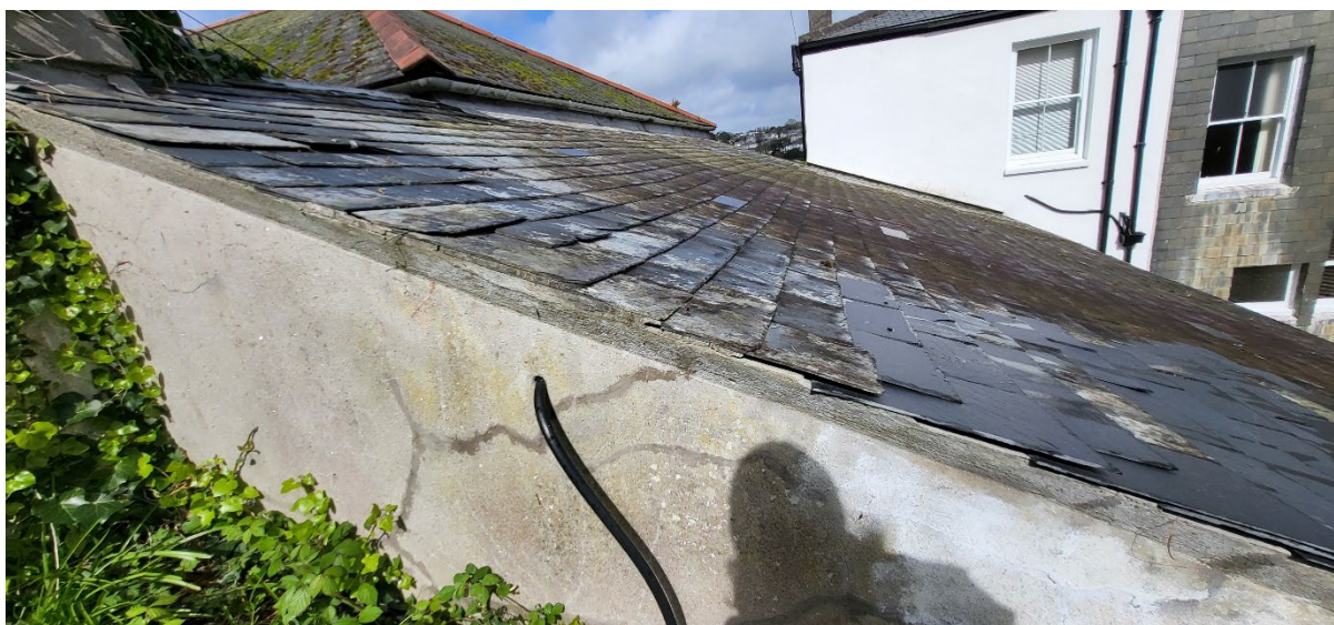
Figure 7: Roof of the annexe with slipped slates and gaps between slates which may provide potential roosting sites for crevice dwelling bats and / or allow access into the interior
