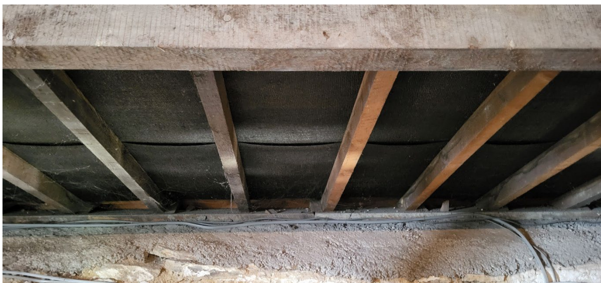
Figure 11: Internal structure of the roof of the annexe (timber lined with bitumen roofing felt)
