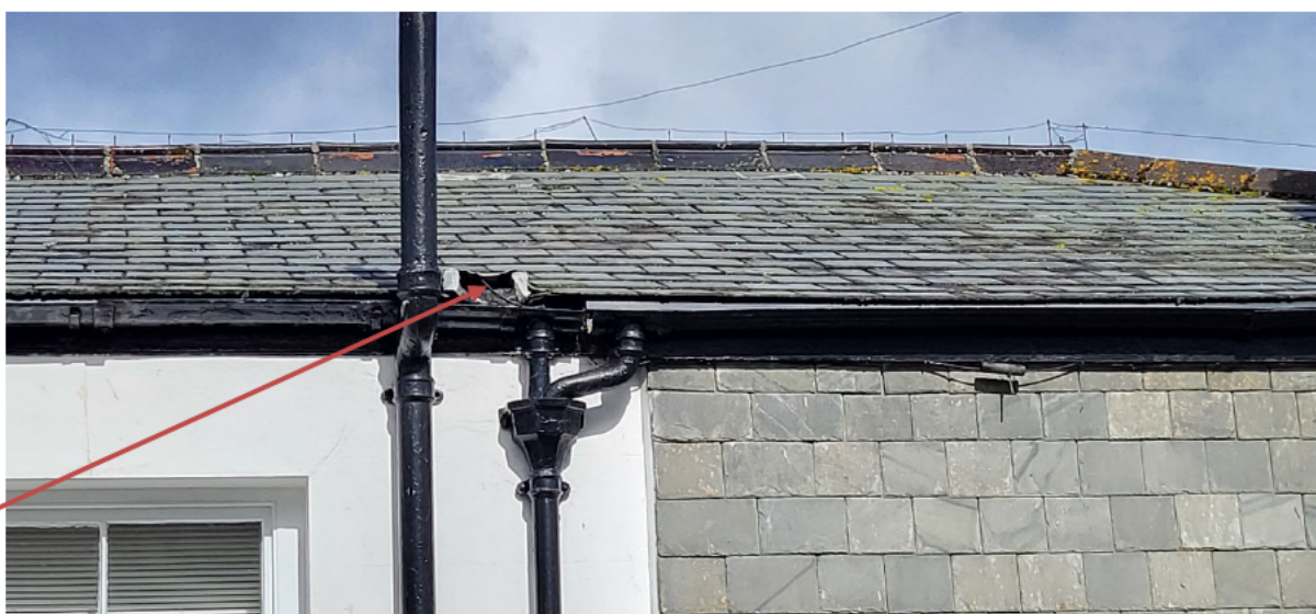
Figure 3: Vent on the roof of the west elevation may provide a crevice for roosting bats and / or access into the roof interior
