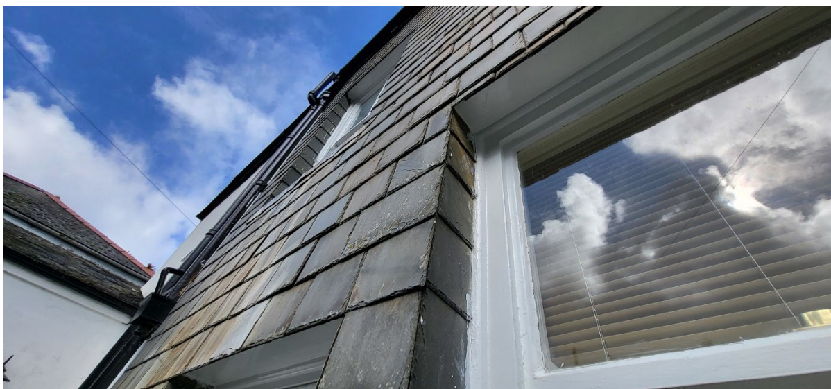
Figure 5: Small gaps behind hanging slates on the west elevation may provide roosting sites for bats
