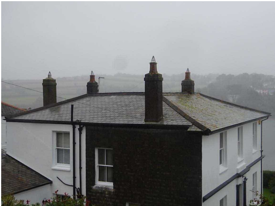
South West and South East facing roof pitches showing location of approved solar panels from within the site boundary and chimney stack to be removed. Note Southerly aspect would cast shadow on solar panels.
