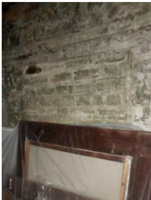
The east wall, blocked up doorway with timber lintel still in position.
