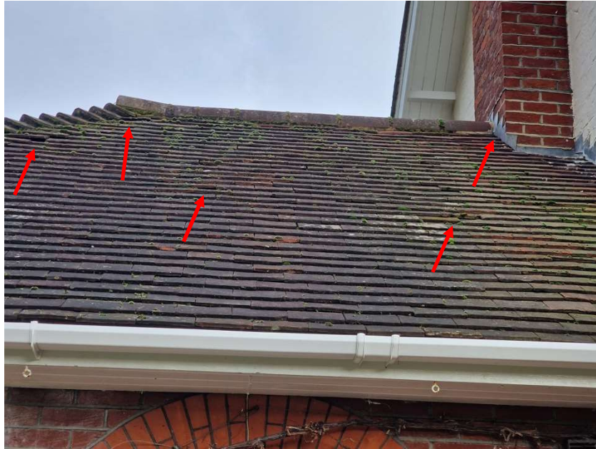
Figure 7. Several lifted concrete roof tiles on the southern elevation (November 2023).
