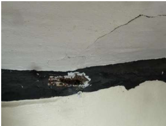
Note :degraded purlin
