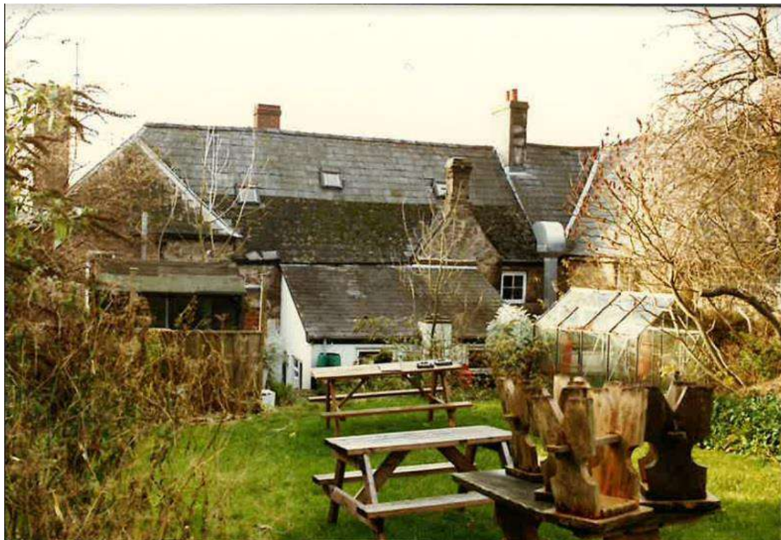
1992 rear from HER ref 232 8/ 63 date 25/ 11/ 92 Buildings At Risk Register
