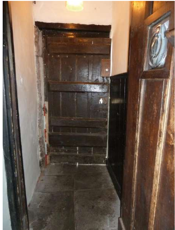
View West of older front door/ dado panelling/ C20 door RH/stone flagstones
