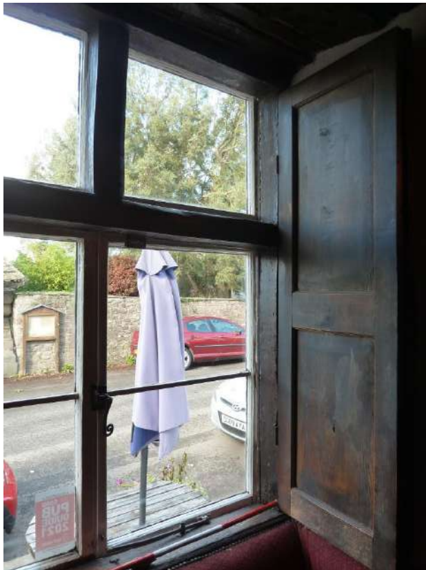
Original timber window frame and transom Inserted C20 casements [Window to corner]
