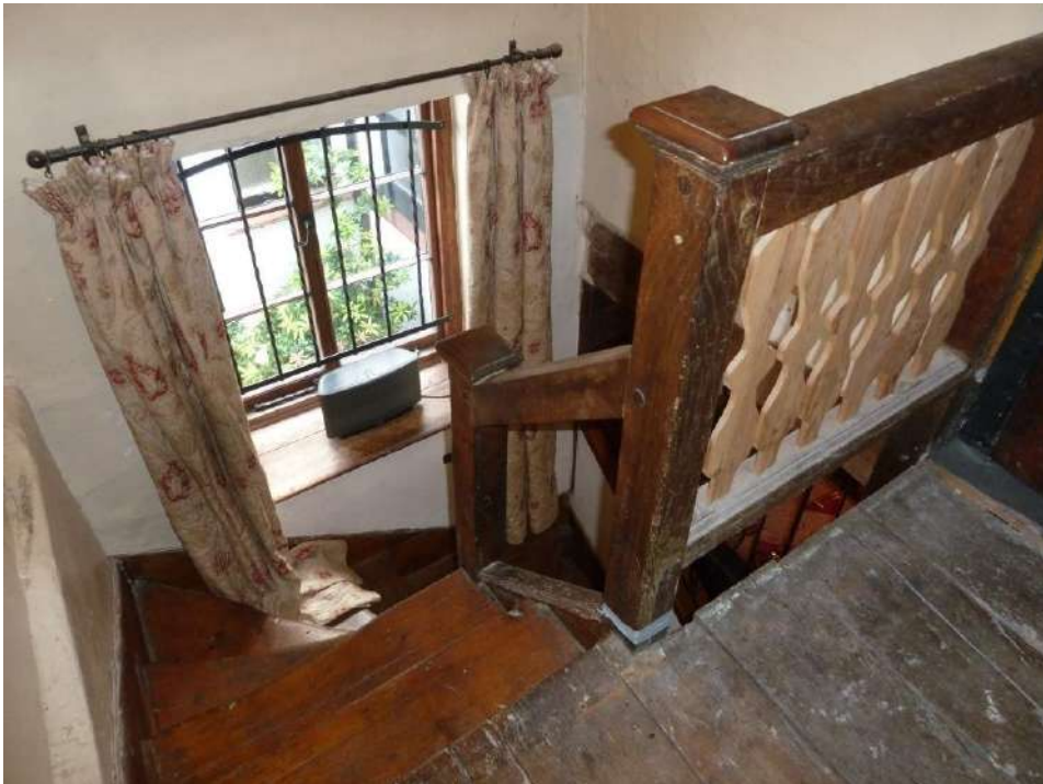
Late C17 oak winder staircase, recent splat balusters of plank have been inserted
