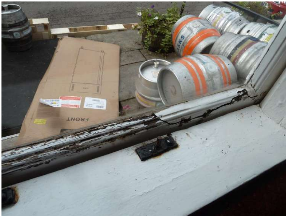
C20 inserted casements poor condition
