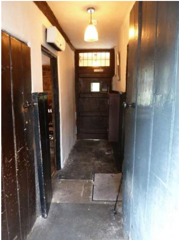
View to West Door to Cellar to LH, Dado Panelling/ C20 inner door/Stone flagstones
