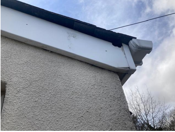
Figure 1 – Hole in kitchen extension barge board
