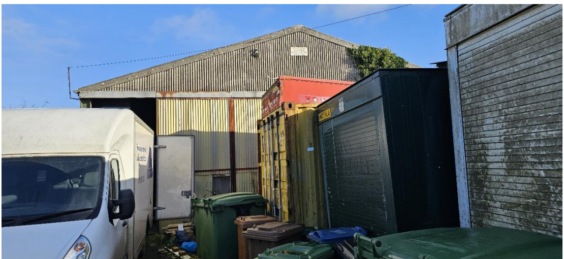
Fig.5: The southwest elevation of the unit proposed for demolition, seen from within the site.
