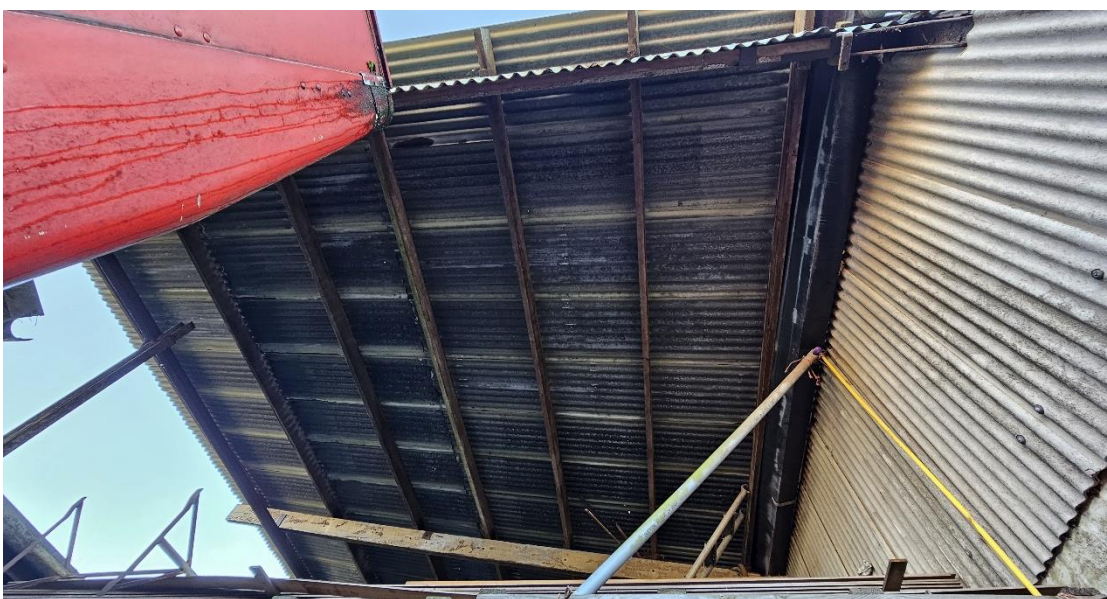
Fig.8: Interior of the unit, constructed of corrugated sheet over a steel frame.
