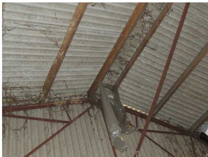
Photo 9: Note cobwebs on walls and roof
