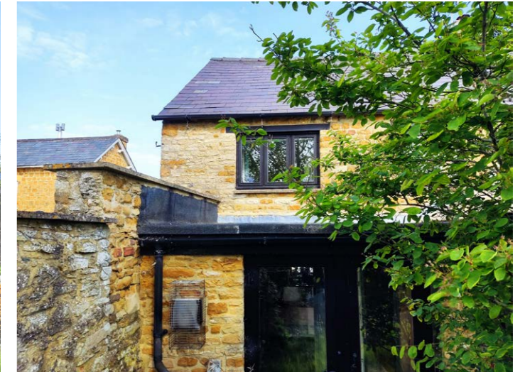
Existing Utility extension attached to boundary wall
