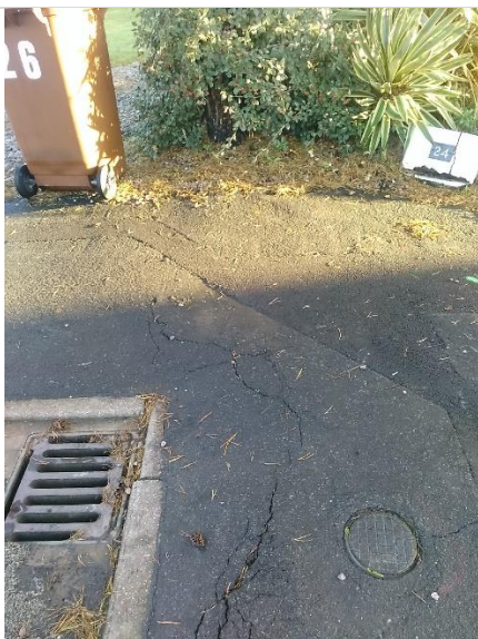
Image 5 – Crack in pavement adjacent to drain to SW of T1
