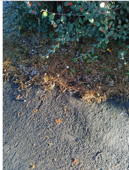
Image 4 – Cracks in pavement to SW of T1
