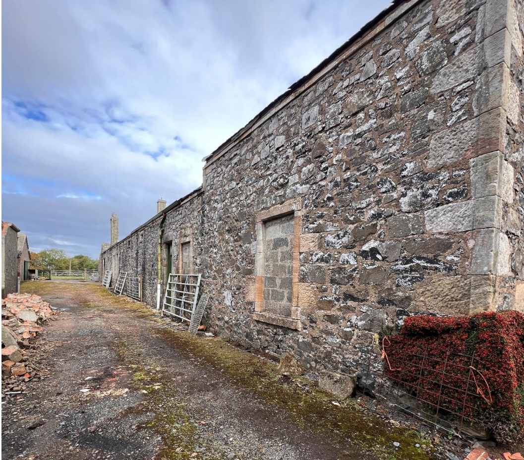
Fig 4: Southernmost corner of the steading showing blocked up window opening.
