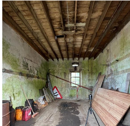
Fig 9: dampness/ water ingress- vegetation growing on walls.
