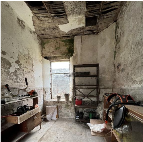
Fig 8: area of ceiling failure/collapse in store
