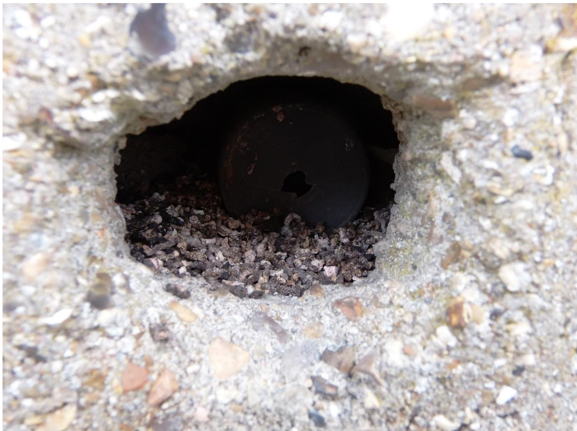
Photo 6 , breezeblock cavity observed on the southern aspect of the building, with approximately 50 droppings indicative of brown long-eared and bird droppings.
