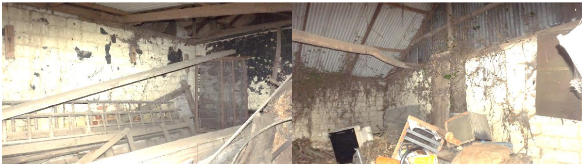
Fig 11 & 12. Internal view of brick, block and clay walls (left) and roof structure (right)
