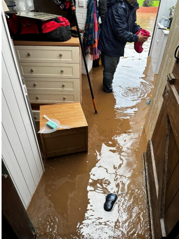
Figure 4.2 Flood water in entrance
