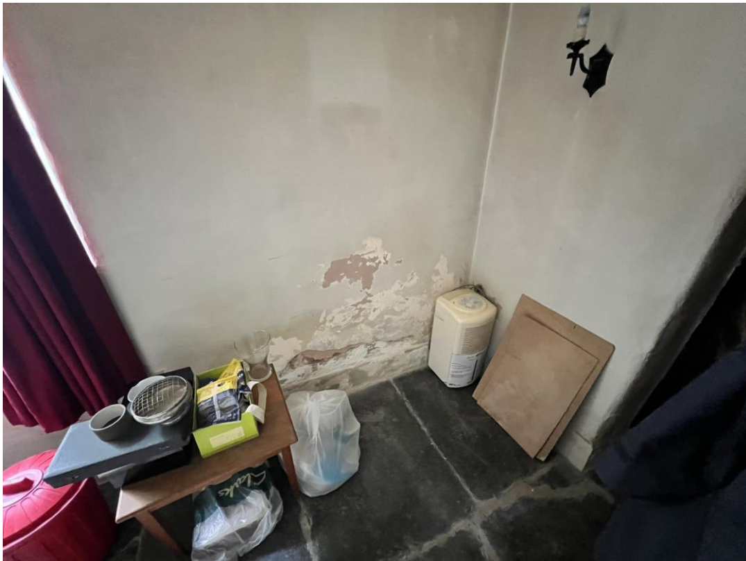
Figure 5 – Photograph showing damp staining and plaster blistering.
