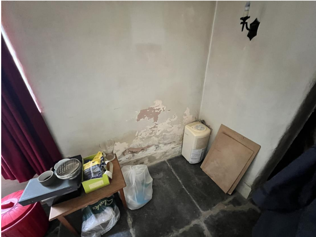
Figure 6 - Photograph showing damp staining and plaster blistering.
