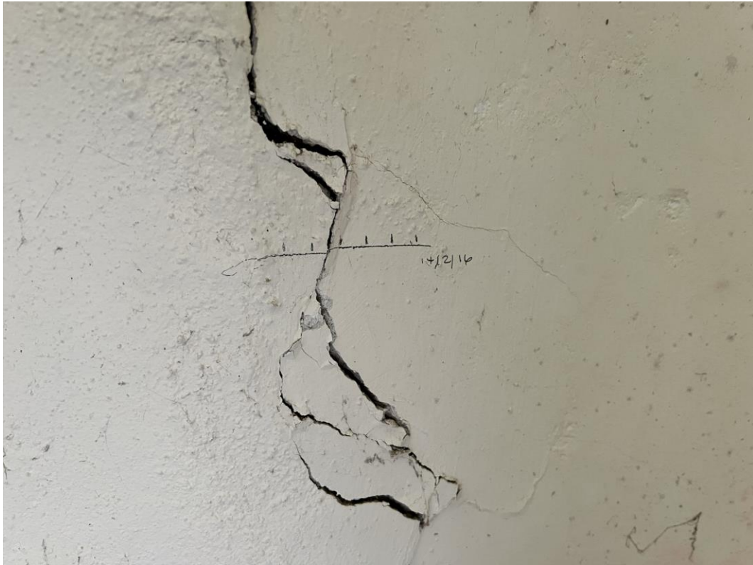
Figure 8 – Photograph showing cracking on first floor landing.
