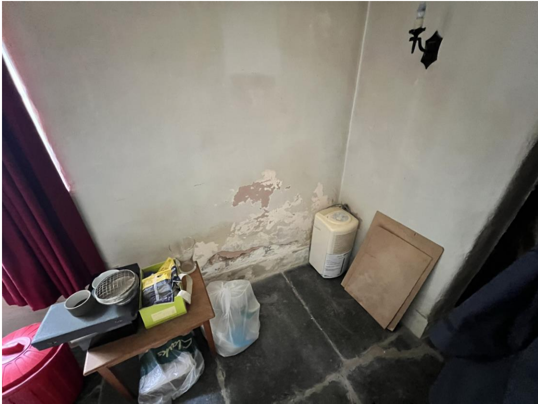
Figure 6 - Photograph showing damp staining and plaster blistering.
