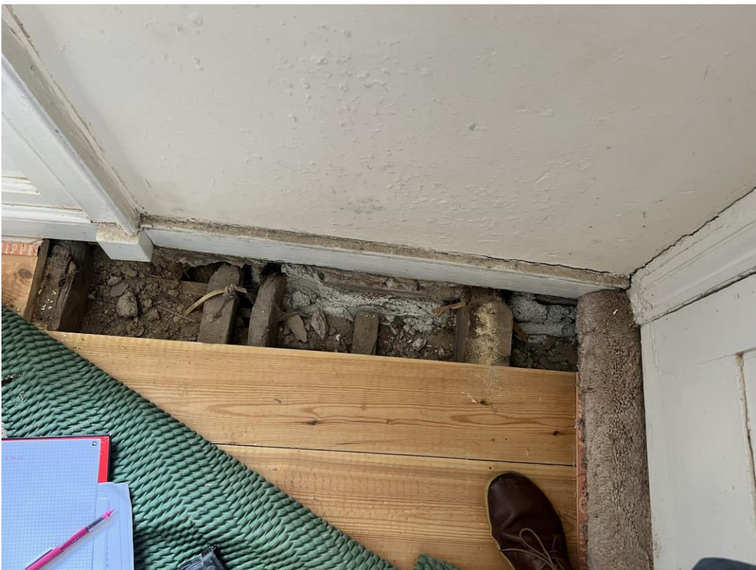
Figure 3 - Photograph showing rotten floor joists to first floor landing.
