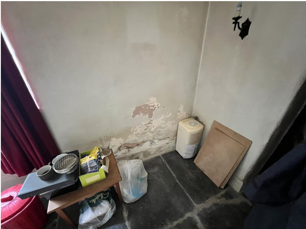
Figure 5 – Photograph showing damp staining and plaster blistering.
