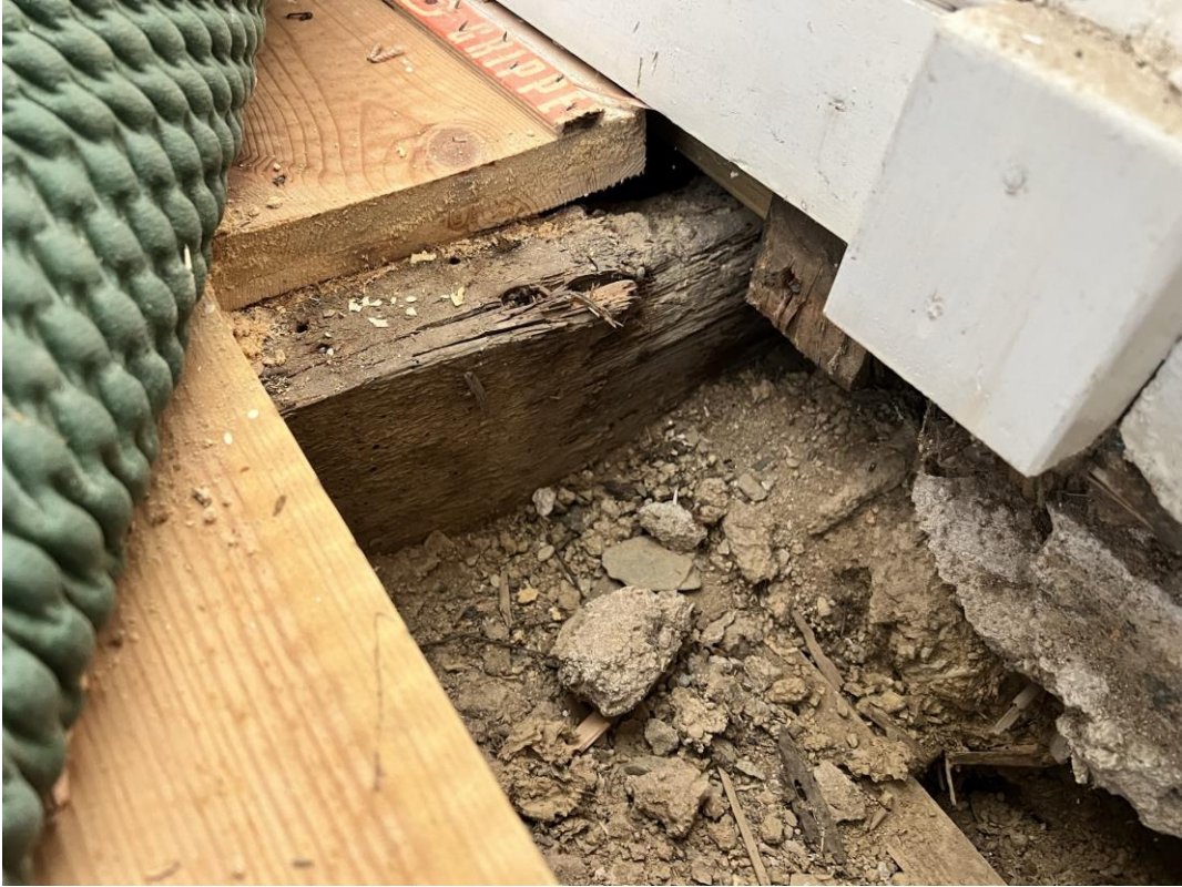
Figure 2 – Photograph showing rotten floor joists to first floor landing.
