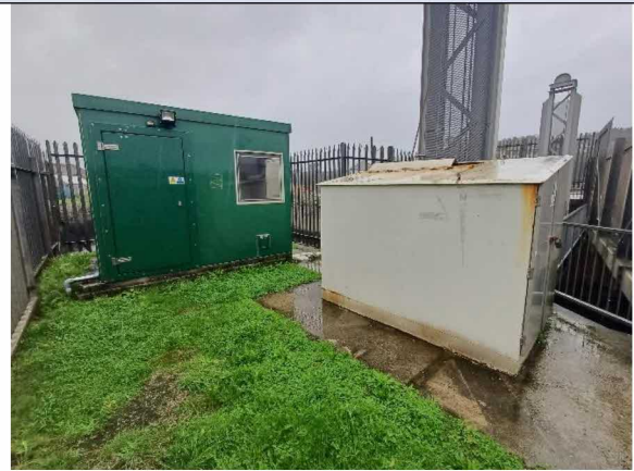
Winch housing to be replaced.
