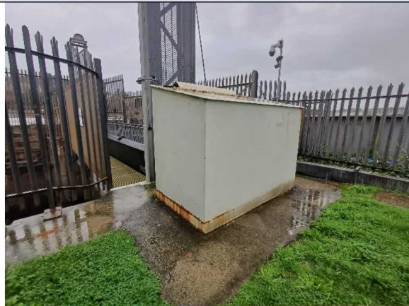
Winch housing to be replaced.
