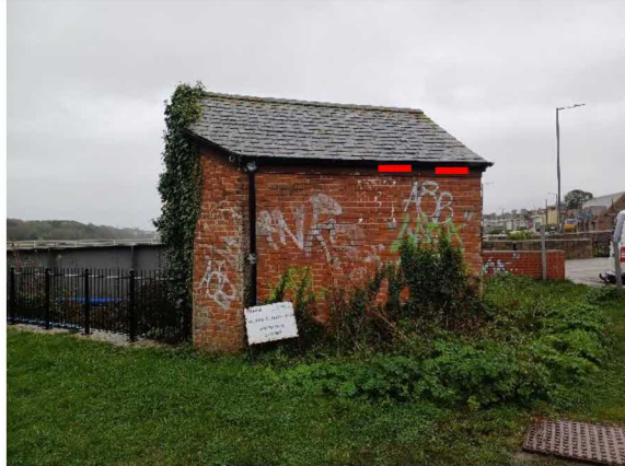
Redundant control building – gaps behind fascia on south-western face.
