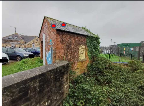
Redundant control building – south-east face and slightly lifted tiles on north-east face.
