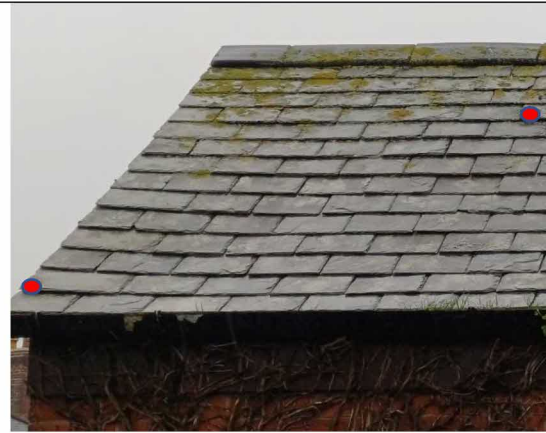
Redundant control building – slightly lifted tiles on north-east face.
