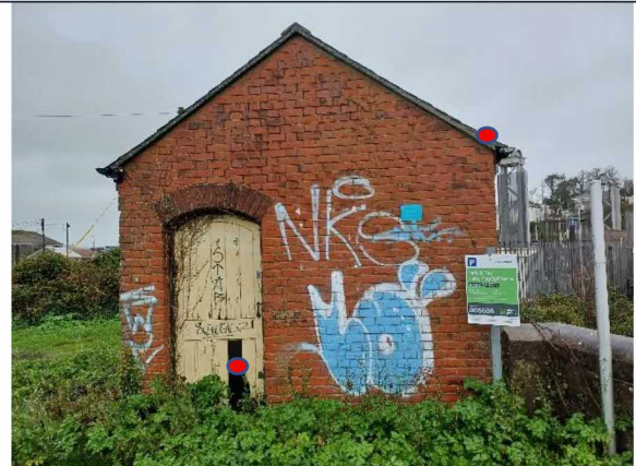
Redundant control building – potential roost access points under lifted tile and through broken doorway on south-eastern face.
