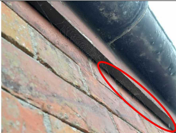
Redundant control building – gap behind fascia in places on south-western face.
