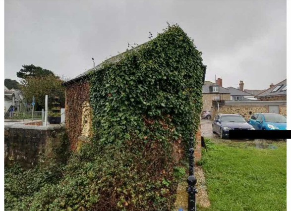
Redundant control building – ivy coverage on north-west face.
