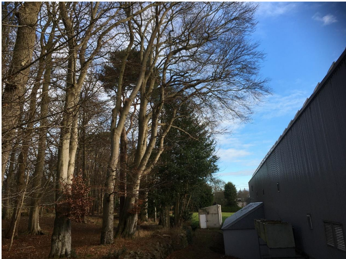
Photo 10 – Mature tree close to rear of sports complex. Includes severely decayed horse chestnut 2482 where removal has been recommended.
