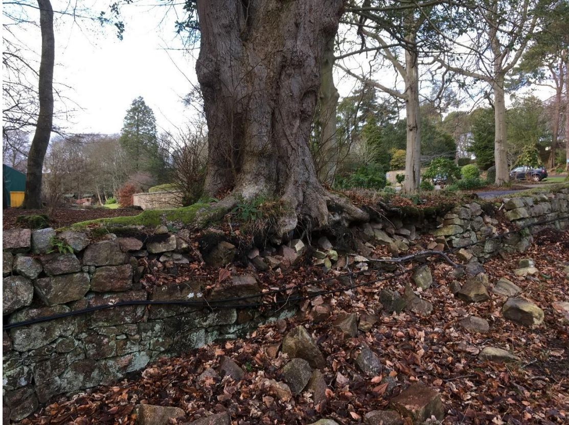
Photo 16 – Large and mature limes 2666, 2668 and 2671 grow from edge of ha ha wall next to driveway. The stone at the base of each tree have fallen from the wall, exposing the roots. The trees are tall with some poorly formed limbs. A 20% crown reduction has been recommended to reduce the risk and encourage the development of a more compact crown.
