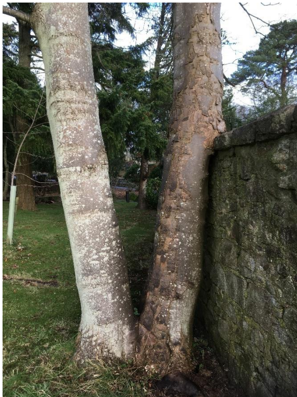
Photo 14 – Twin stemmed sycamore 2633. Co-dominant stem should be removed to protect wall.
