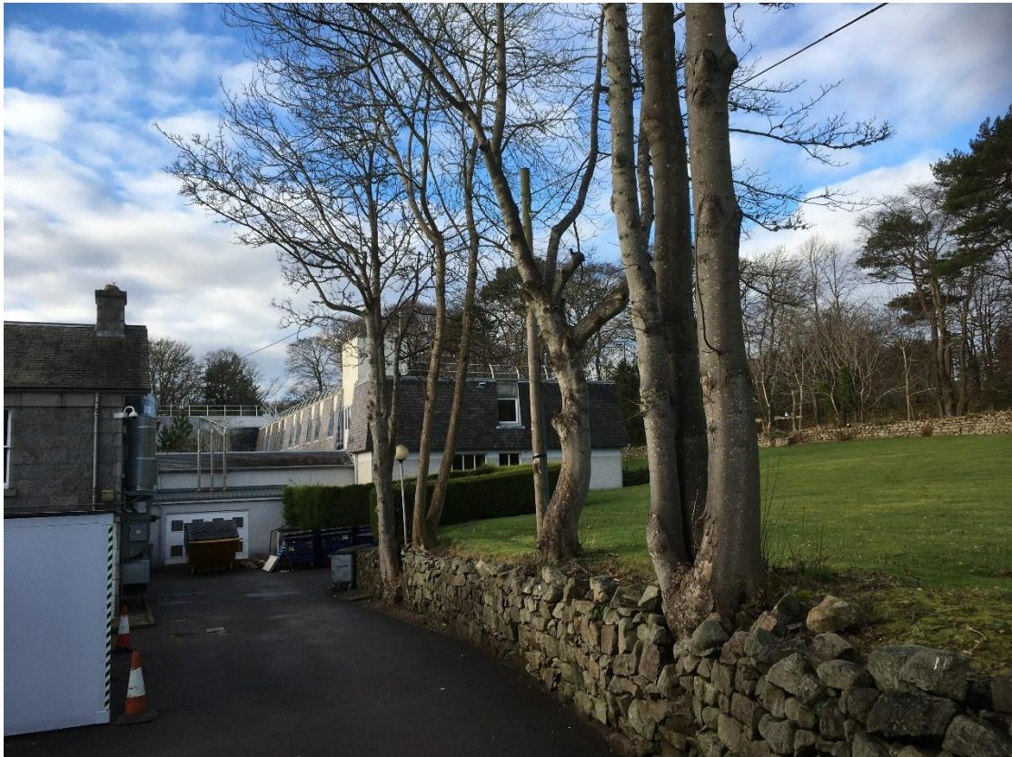
Photo13 – Semi mature trees 2595 to 2598 growing from wall and displacing stones.
