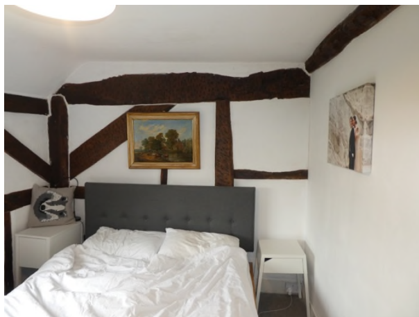
Figure 21: Later partition subdividing the first floor space and timber framing with straight head braces
