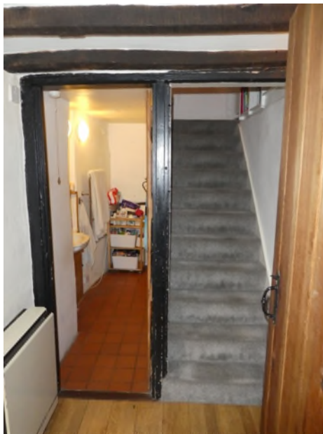
Figure 13: Likely position of the original stairs to the rear of the existing stairs
