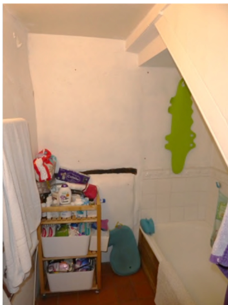
Figure 14: Possible blocked opening between 1 and 2 The Close (bathroom)
