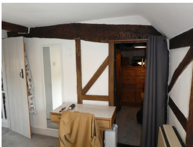
Figure 19: Chimney breast with cupboard to the right in the main bedroom on the first floor
