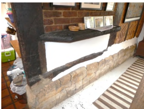
Figure 10: Sill for an oriel window on the original north-west elevation viewed from the dining room
