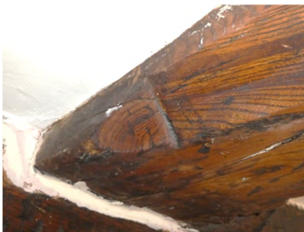
Figure 20: Detail of the chamfered beam with scroll stops on the first floor
