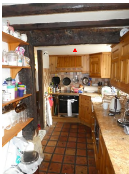
Figure 17: Cross beam with mortices along the soffit demonstrating a removed section of timber frame and stone plinth
