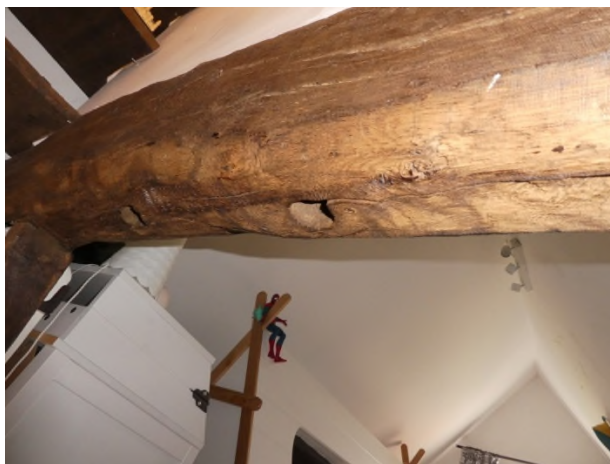
Figure 23: Stave holes for a wattle and daub panel over the door to the attic bedroom
