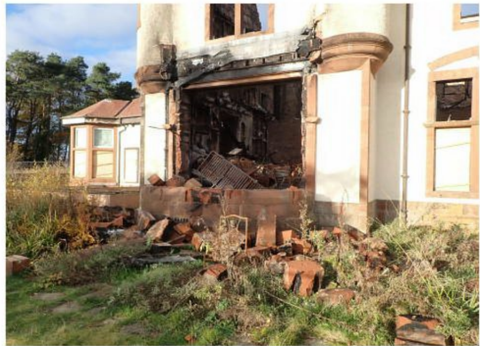
Photograph 2: Taken on the southwest facing elevation looking onto the window opening to the former conferencing suite shows the masonry that collapsed suddenly in early September.
