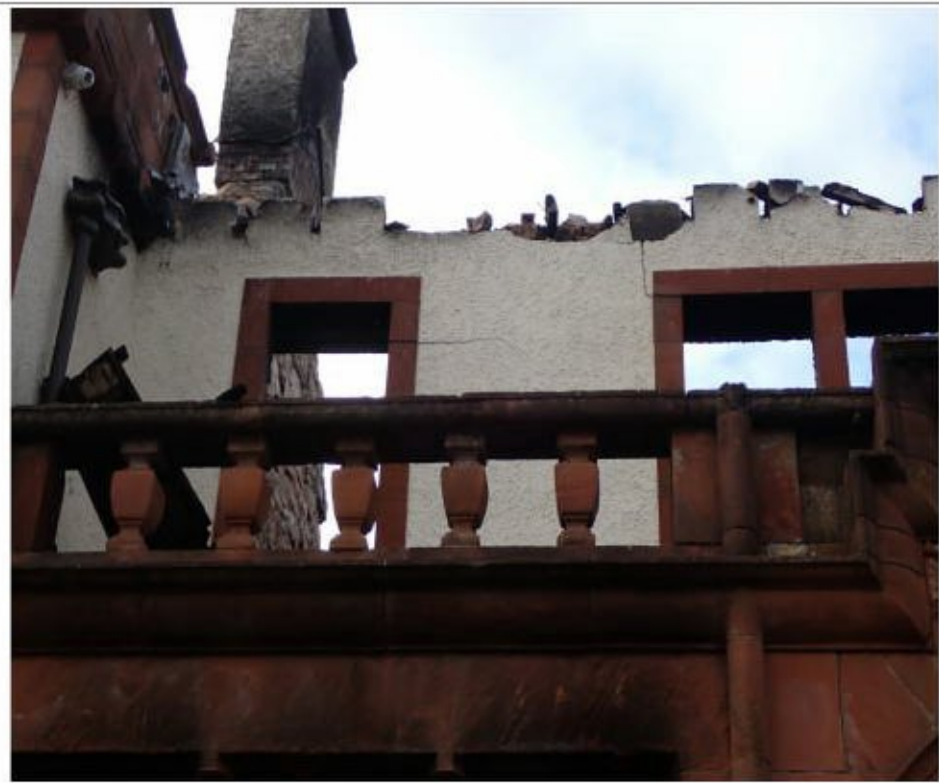
Photograph 4: Taken on the southeast facing elevation looking onto the wall panel directly above the red sandstone arched main entrance to the former hotel. Note the cracking that emanates from the lintels of both windows.
