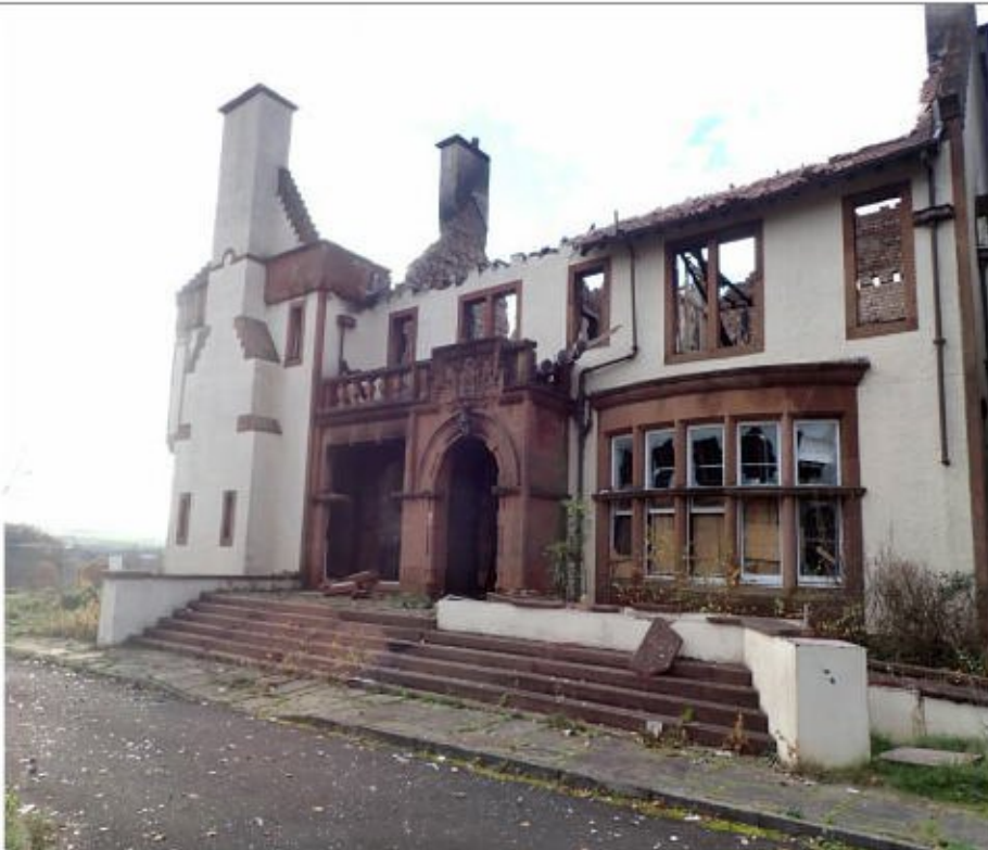
Photograph 3: Taken on the southeast facing elevation looking onto the red sandstone arched main entrance to the former hotel.
