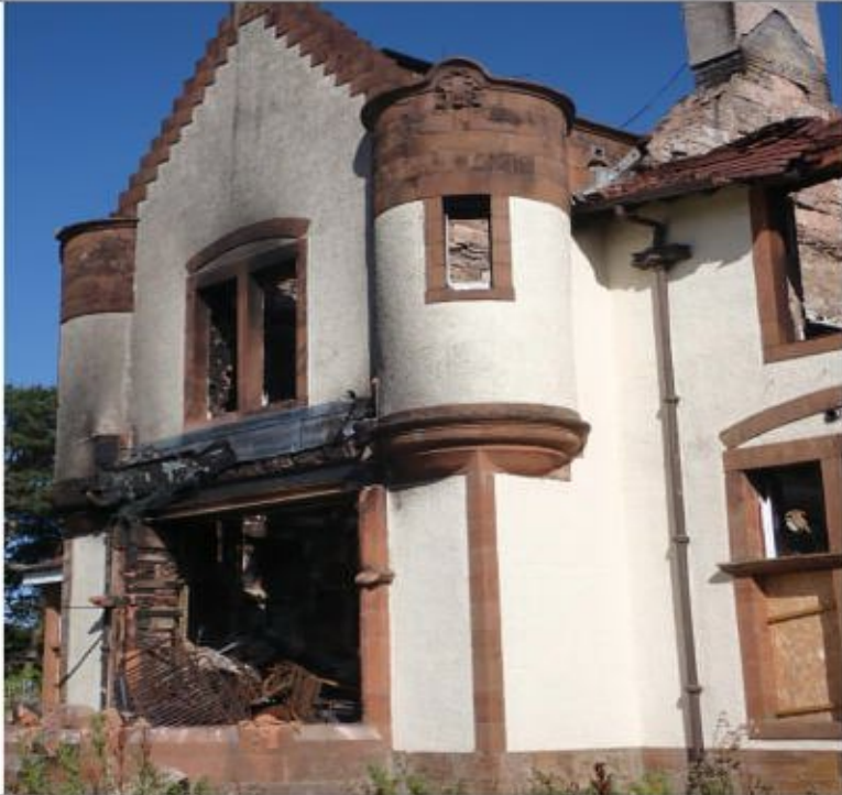
Photograph 1: Taken on the southwest facing elevation looking onto the window opening to the former conferencing suite.
