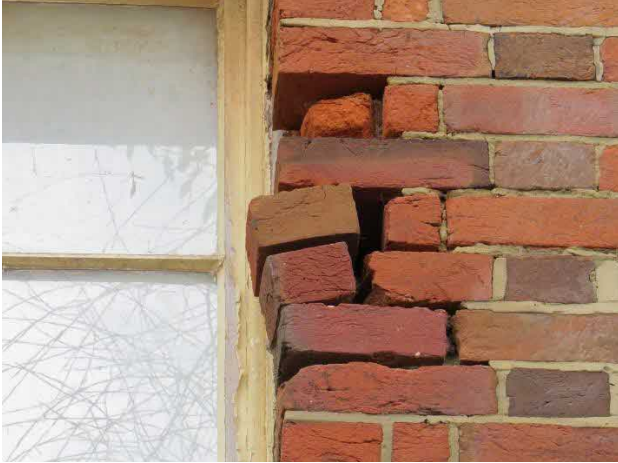
Photo 1. An example of the damaged brickwork on the building.
