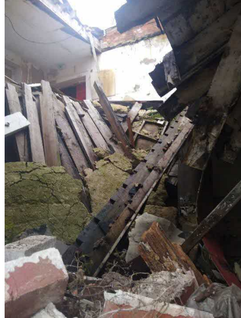
Photo 2. The section of roof that has collapsed.
