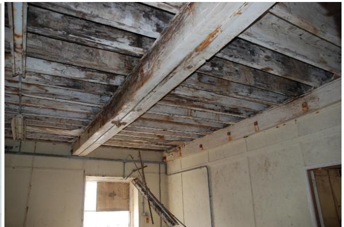
Partially collapsed roof in 2023
