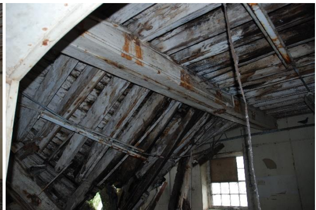
Collapsed roof in 2023
