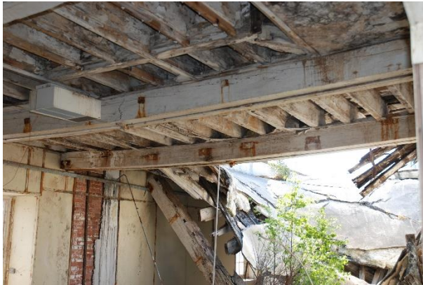
Collapsed roof in 2021
