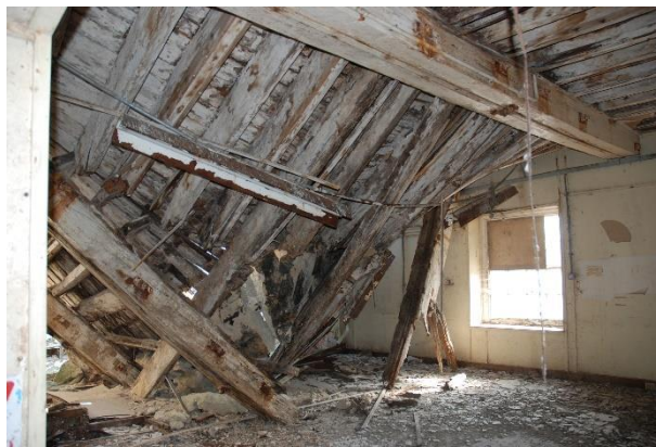
Collapsed roof in 2021
