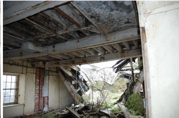
Collapsed roof in 2023
