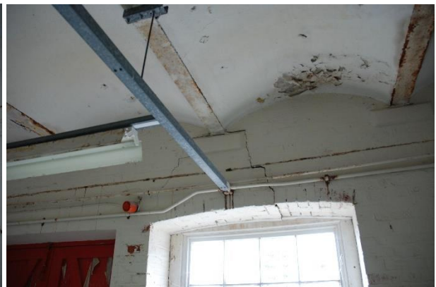
Crack over window in 2023
