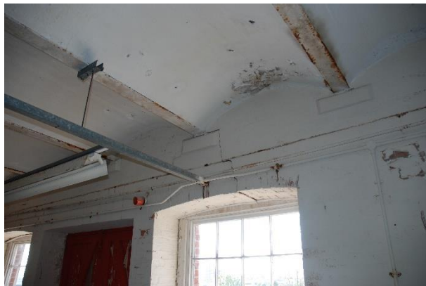
Crack over window in 2021
