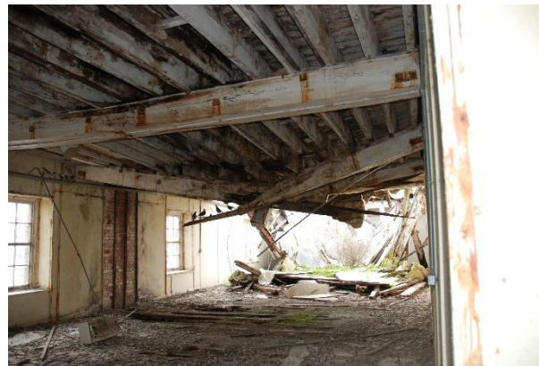
New collapse in 2023
