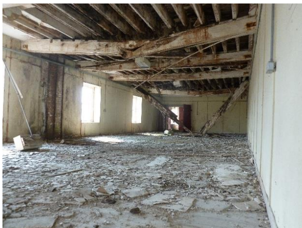
Partially collapsed roof in 2021
