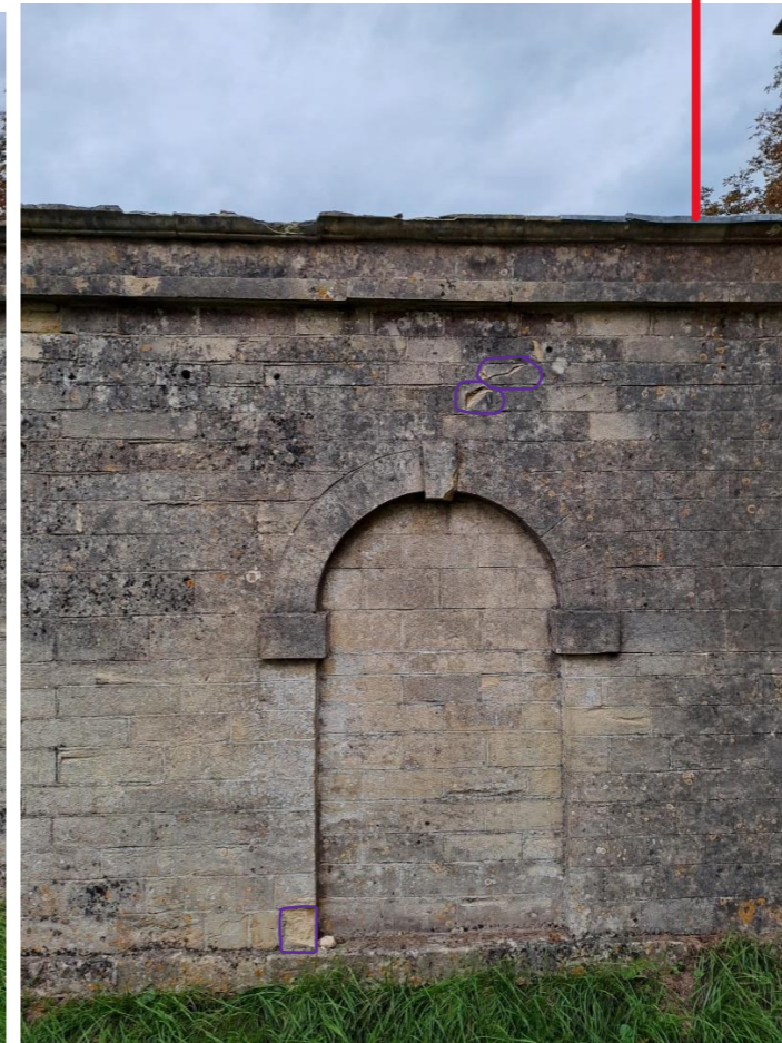
Mortar repairs to upper face of lower copings to prevent water ponding
