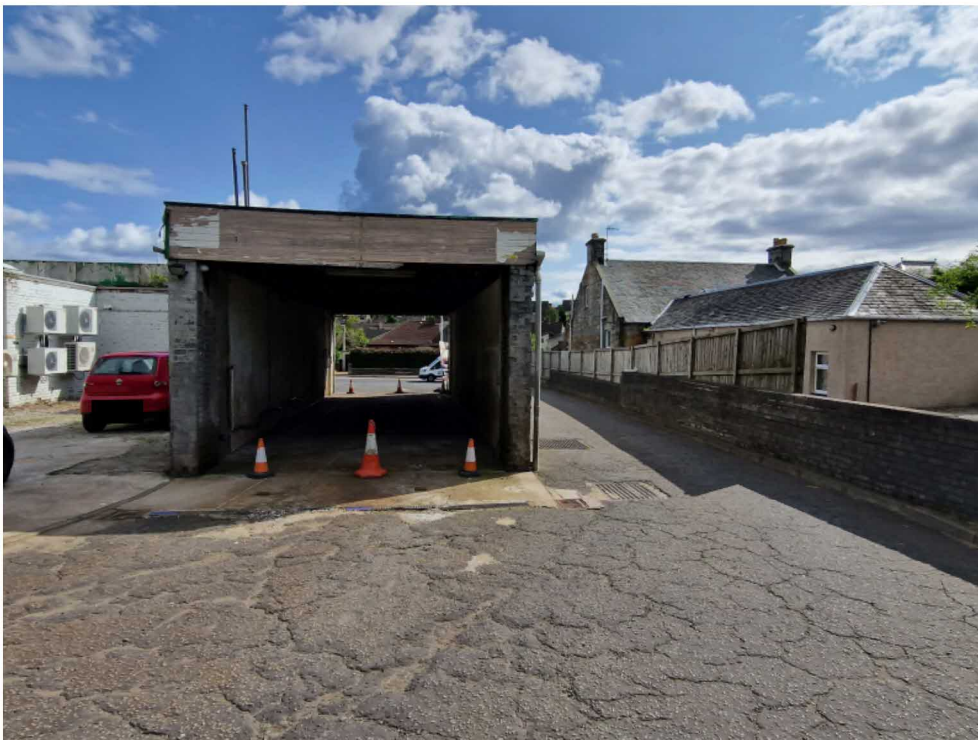
Figure A1.4: As Figure 1.3 but with view of missing fencing section and ground floor window to rear of 82 Halbeath Road
