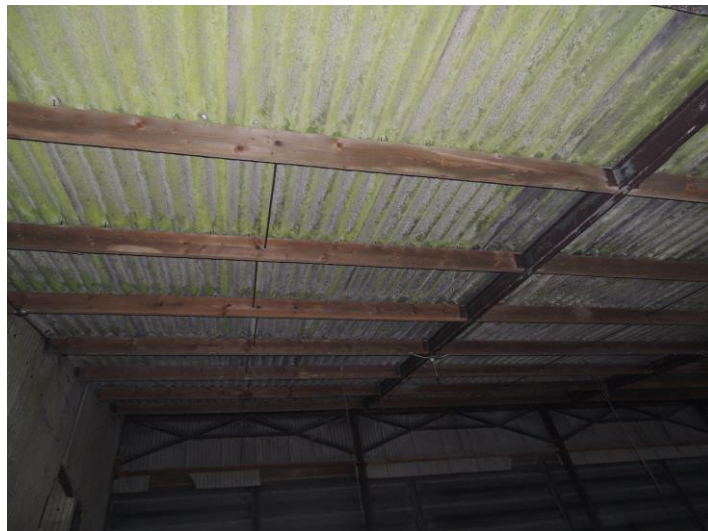
Photo 7: The roof of the store had no features that might be occupied by bats
